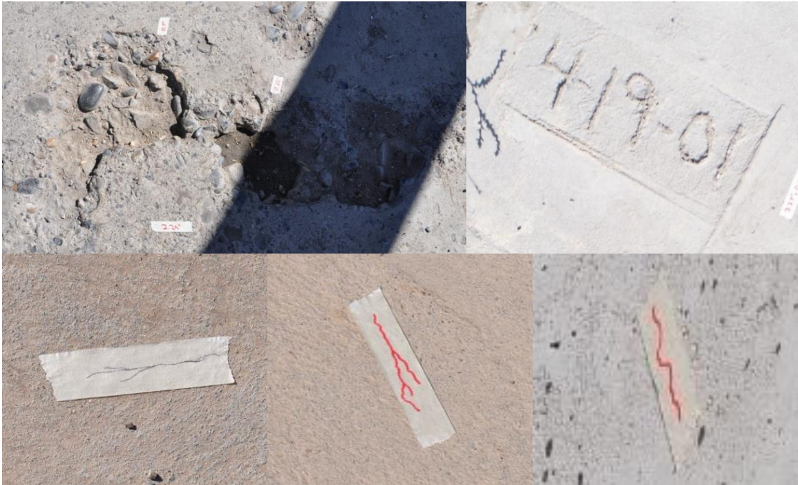
Figure 90. Defects in the Trenton and Elwood Bridges; Defect 1: a pothole (top left); Defect 2: a numeral 1 (top right); Defect 3: a pen-drawn crack (bottom left); Defect 4: a marker-drawn crack (bottom center); Defect 5: a marker-drawn crack (bottom right).
