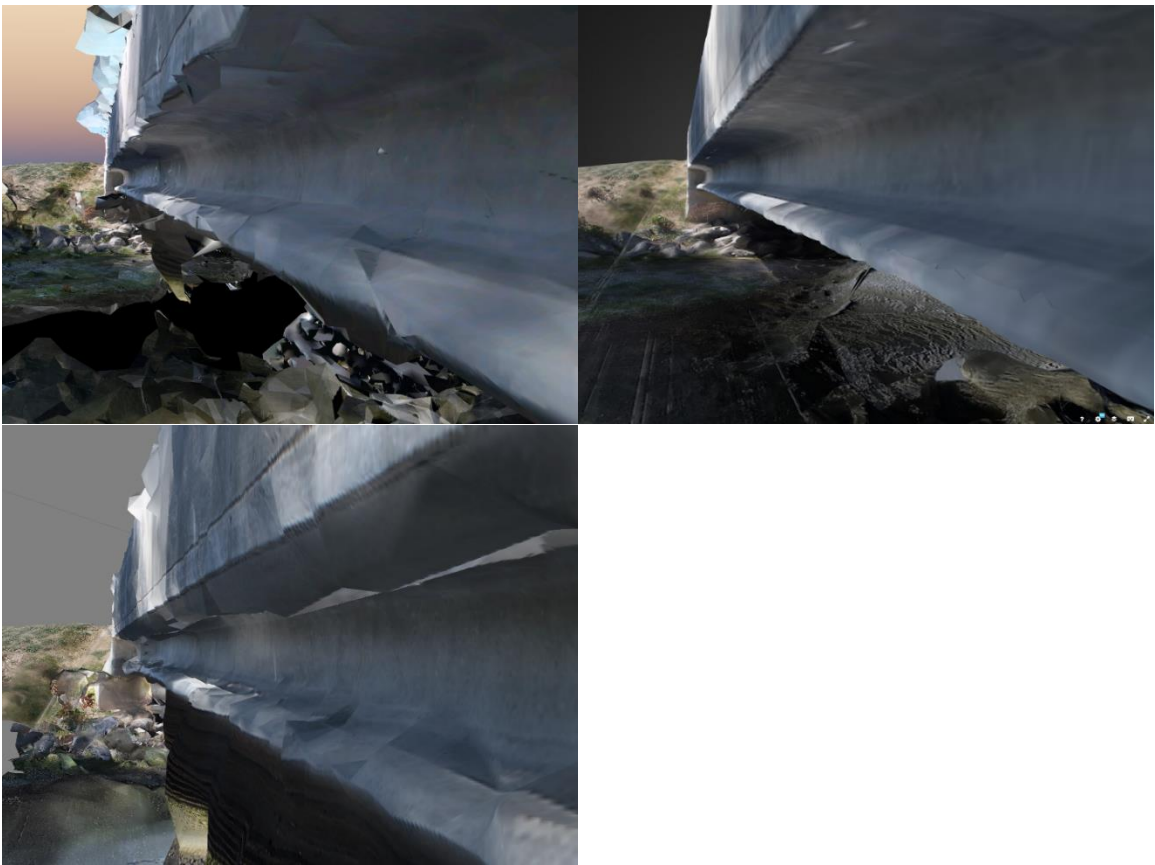
Figure 80. Screenshots of Girder 10 from the Pix4D (top left), DroneDeploy (top right), and Agisoft PhotoScan (bottom left) Nibley Bridge models.
