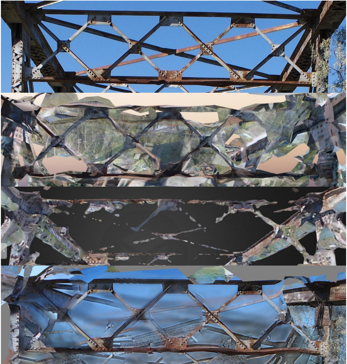
Figure 82. Trenton Bridge sway bracing from a drone photograph (top) the Pix4D (top center), DroneDeploy (bottom center), and Agisoft PhotoScan (bottom) models.
