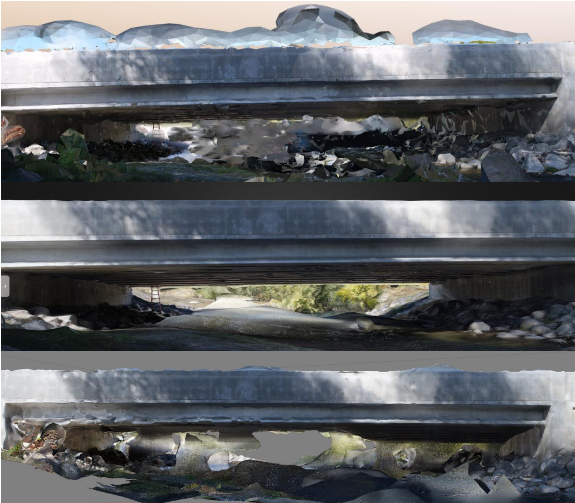
Figure 78. Screenshots of the underside of the Nibley Bridge Pix4D (top), DroneDeploy (center), and Agisoft PhotoScan (bottom) models.
