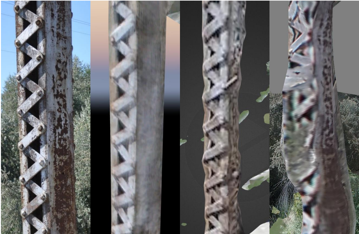
Figure 85. Photograph of a Trenton Bridge vertical truss member (left) compared against screenshots of the Pix4D (center left), DroneDeploy (center right), and Agisoft PhotoScan (right) models.
