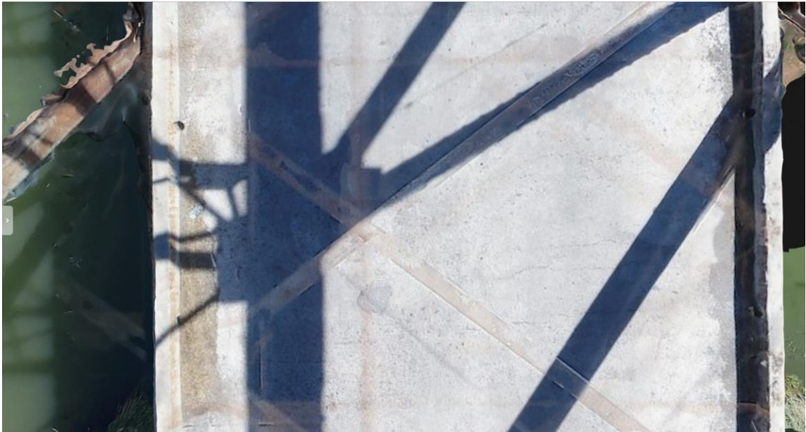
Figure 84. “Phantom” image of the top lateral bracing from the DroneDeploy Trenton Bridge model.
