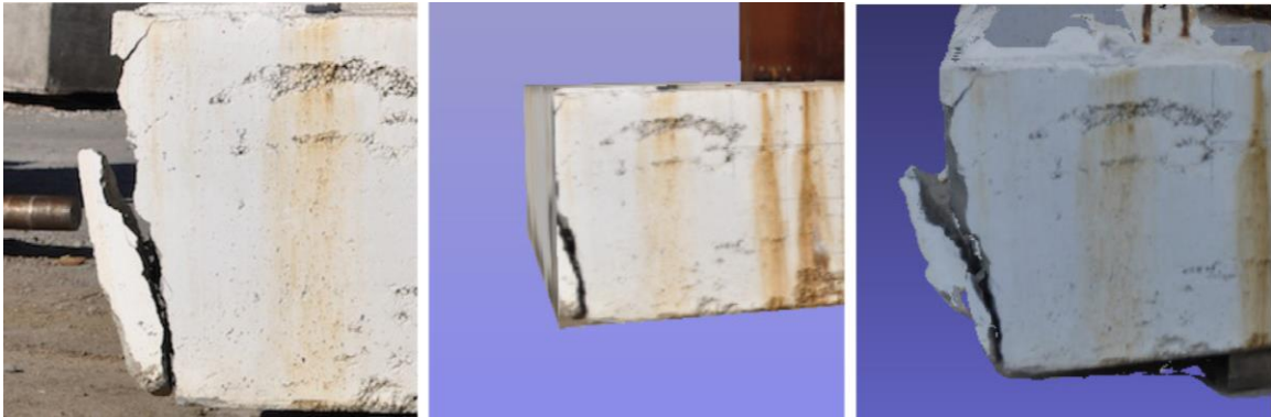
Figure 7. Spalling on the column (left), IM model (center), and DSfM model (right) (Lattanzi and Miller 2015).
