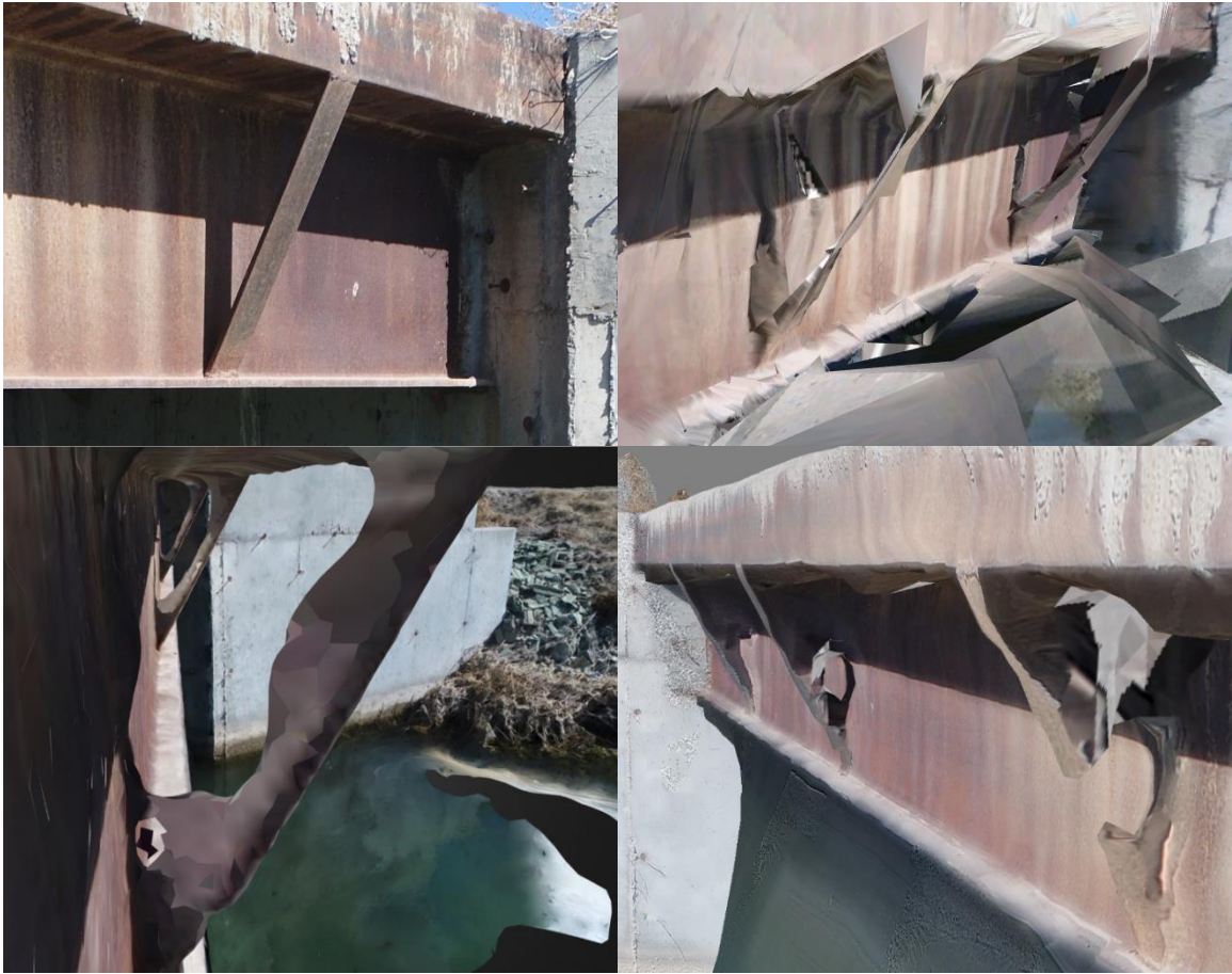
Figure 89. Photograph of the Elwood Bridge flange bracing (top left) compared against screenshots of the flange bracing from the Pix4D (top right), DroneDeploy (bottom left), and Agisoft PhotoScan (bottom right) models.
