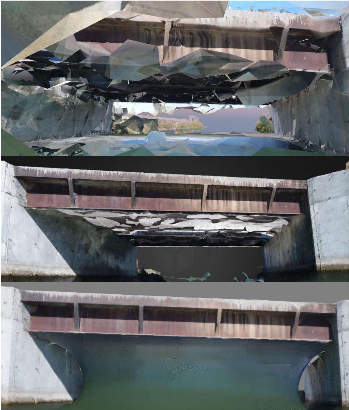
Figure 88. Screenshots of the underside of the Elwood Bridge Pix4D (top), DroneDeploy (center), and Agisoft PhotoScan (bottom) models.
