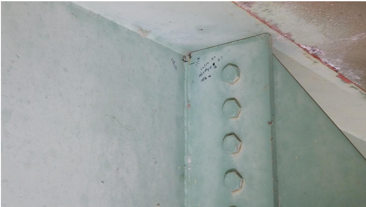
Figure 58. Defect (Crack) on the Fourth Floor Beam, Southern Corner, E032
