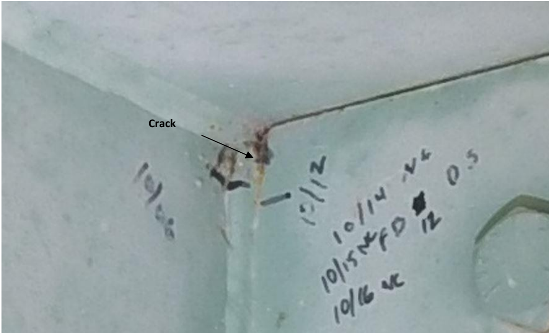
Figure 59. Zoomed Image from the Fatigue Crack on the Fourth Floor Beam, Southern Corner, E032
