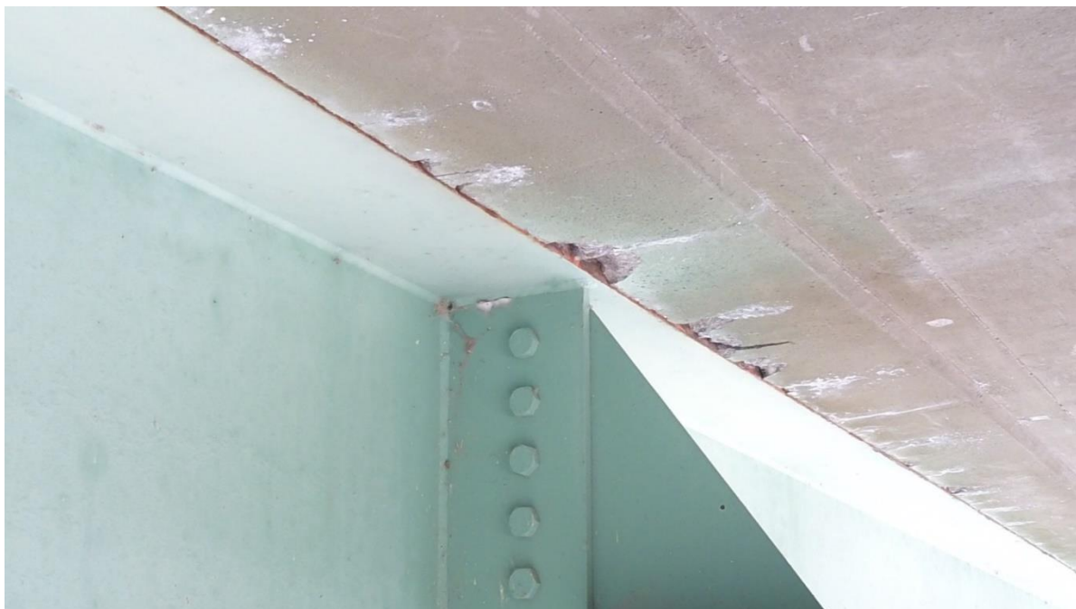
Figure 54. No Cracks on Second Floor Beam on East, Southern Corner, Minor Deck Spalling, E024
