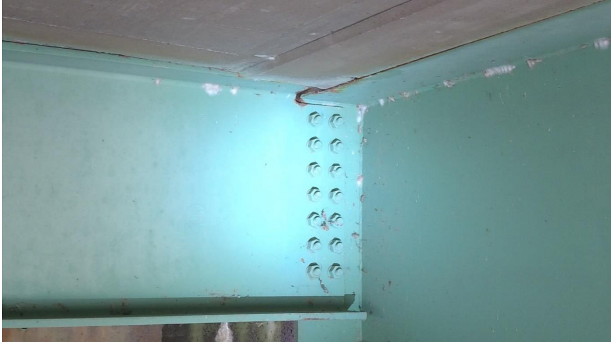
Figure 52. First Floor Beam on East, Southern Corner, Debris on the Weld, E022
