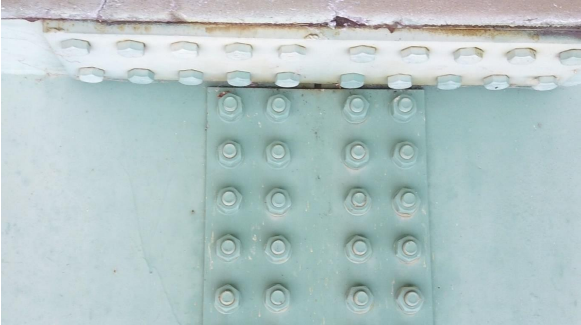
Figure 61. Minor Corrosion on Top of the Northern Girder Splice (First Splice from East), E033
