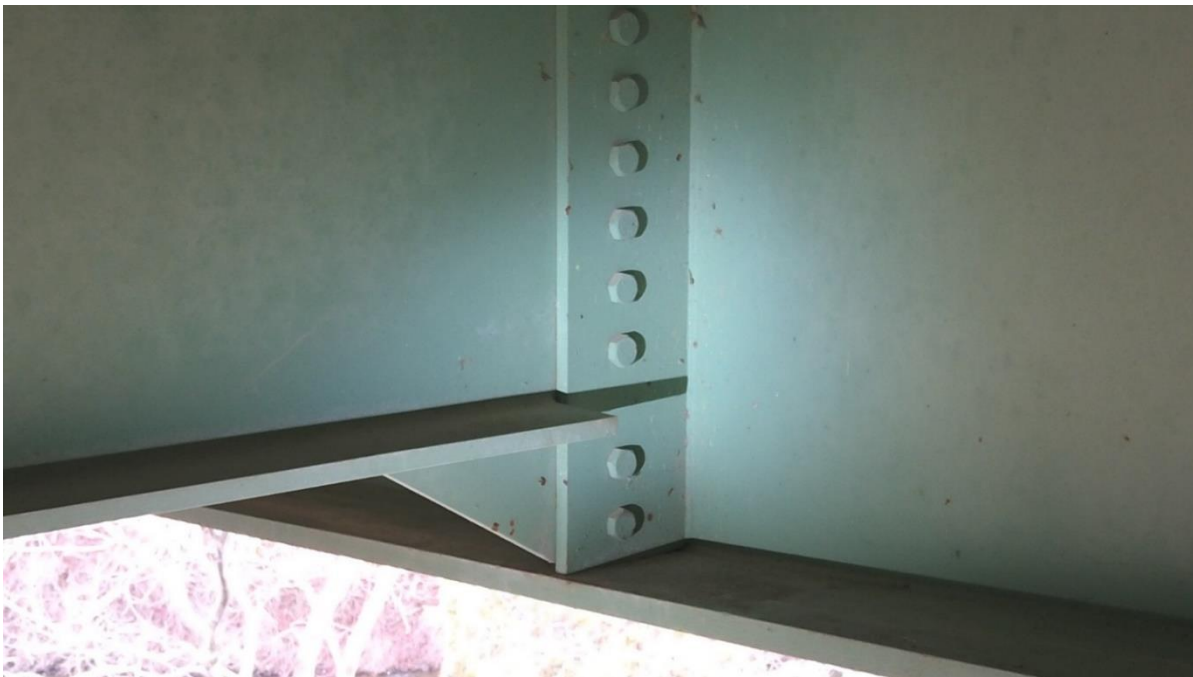
Figure 53. No Cracks on Second Floor Beam on East, Southern Corner, E023
