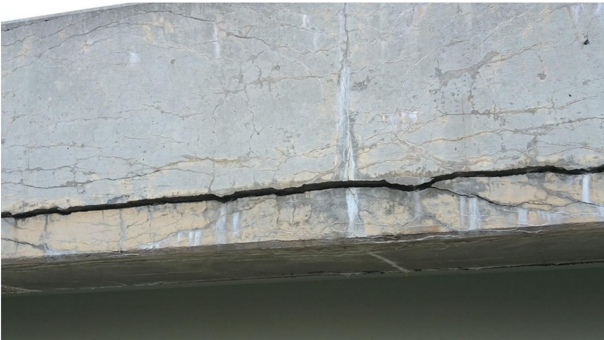
Figure 64. Cracks and Possible Delamination on the Southern Barrier, E036
