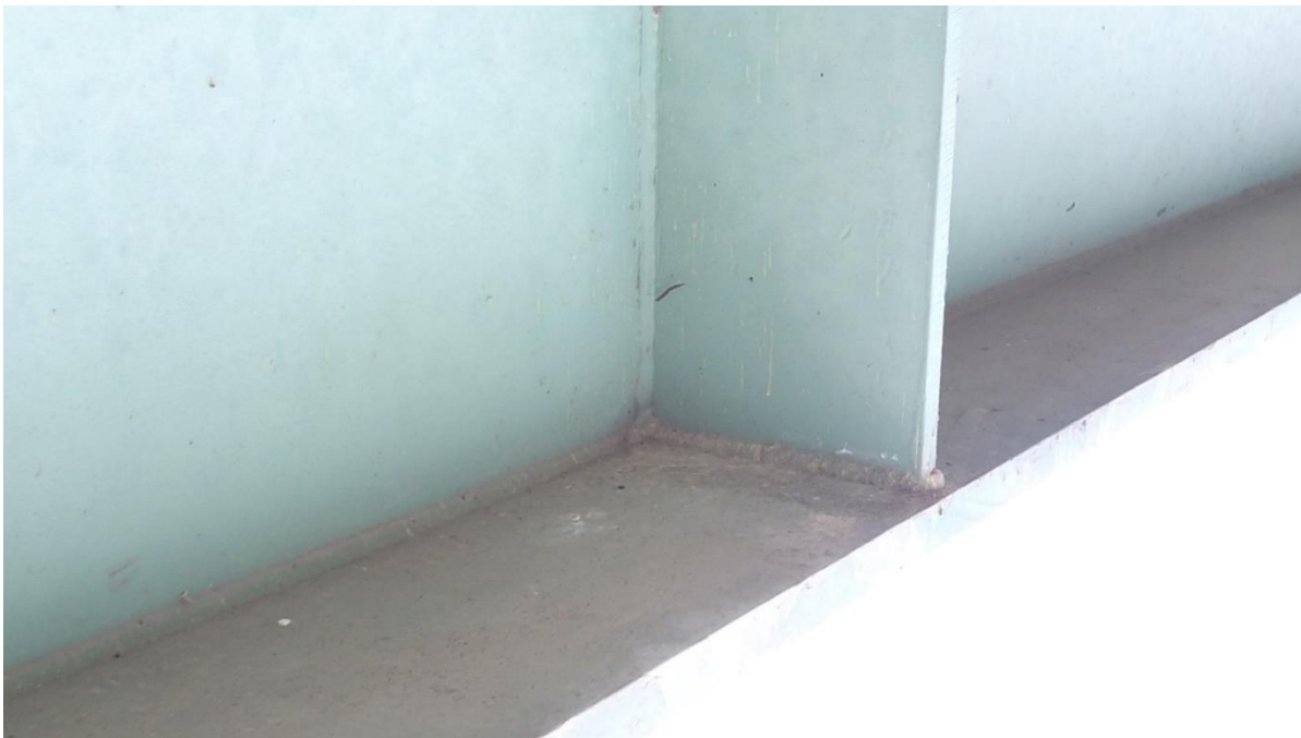
Figure 60. No Defects (Crack) on the Fourth Floor Beam, Southern Corner, Bottom Flange Weld, E032
