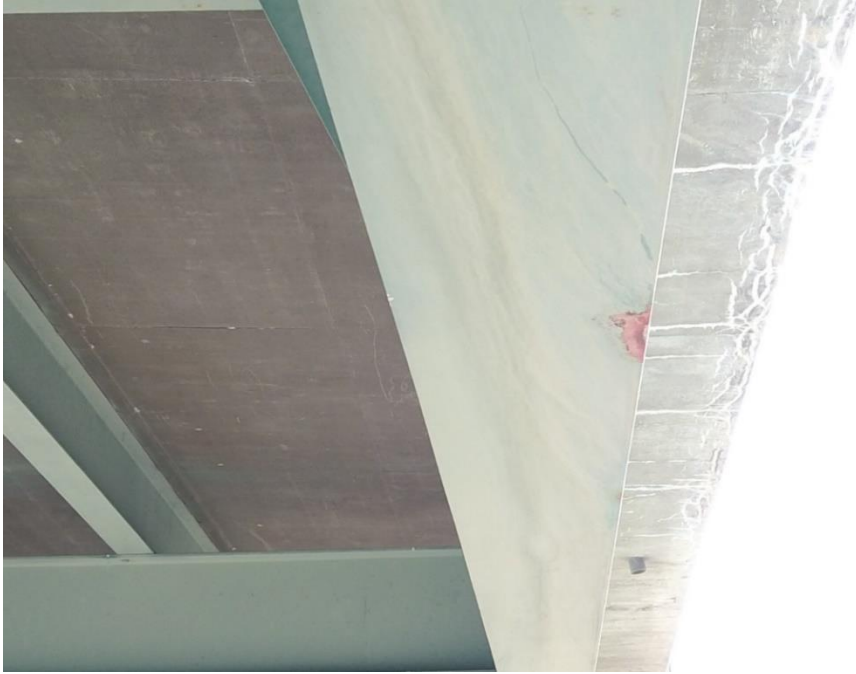
Figure 65. Minor Corrosion on Bottom Flange of the Southern Girder, E035 and E036
