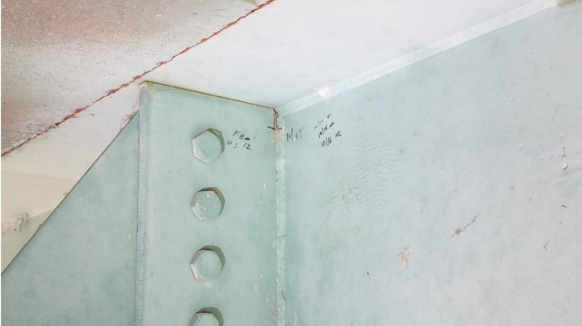
Figure 56. Defect (Crack) on the Fourth Floor Beam, E031
