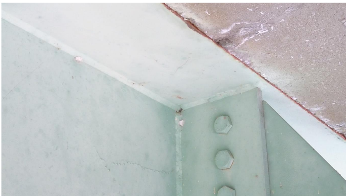
Figure 55. Third Floor Beam on East, Mild Rust, Northern Corner, E027
