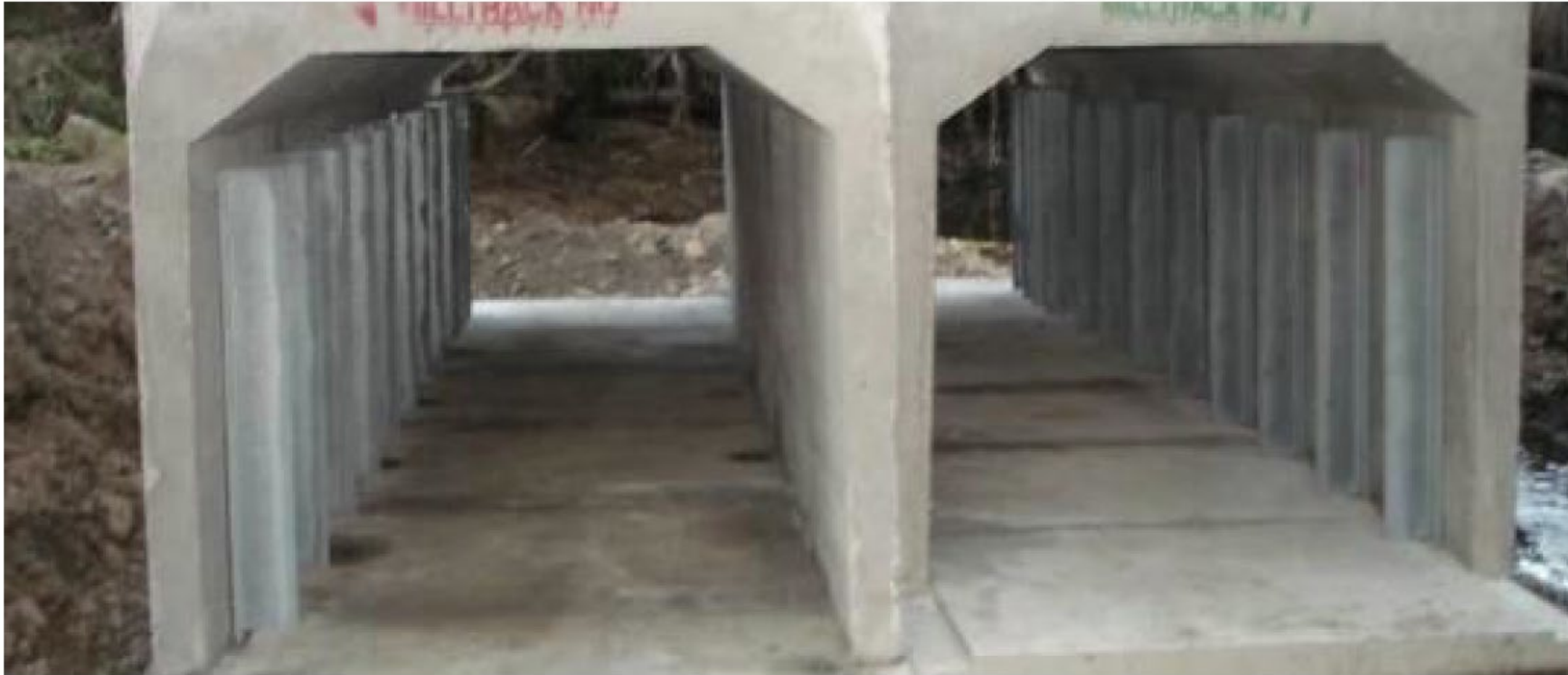
Figure 3.5: Box culverts fitted with single-sided baffles.
