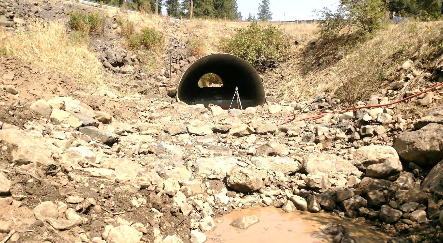
Big Meadow Creek Culvert - Pre Project Conditions
