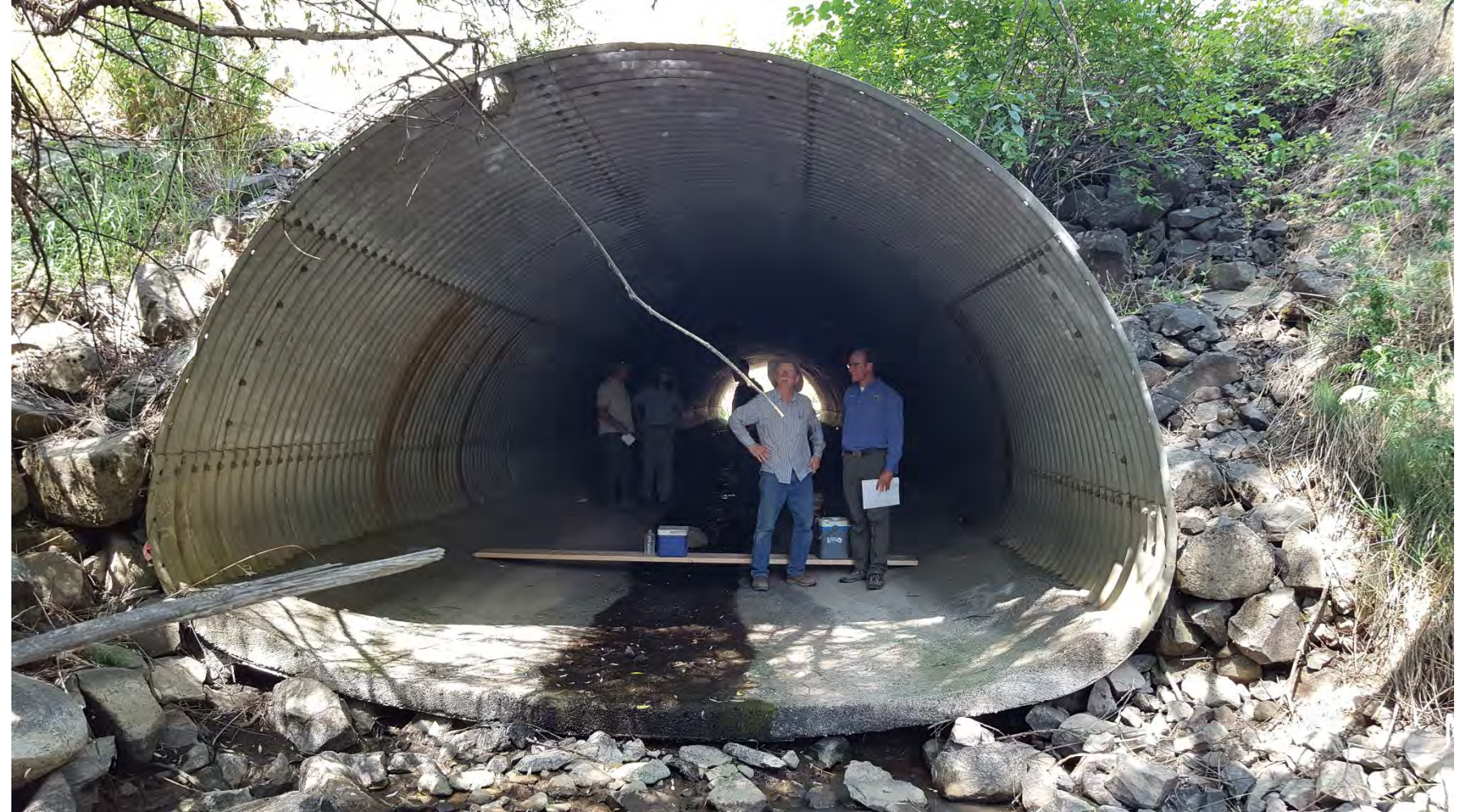
Big Meadow Creek Culvert Pre-Project Conditions
