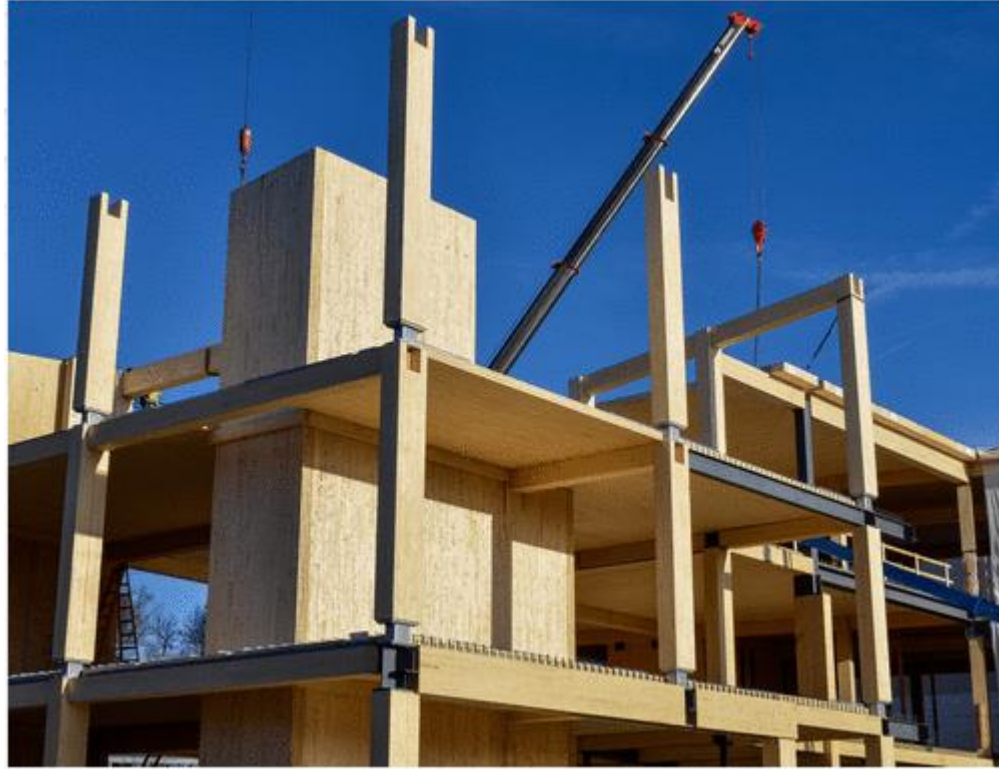
Figure 1.5. The John W. Olver Design Building at the University of Massachusetts under Construction in May 2016 (Photo credit: Alexander C. Schreyer)
