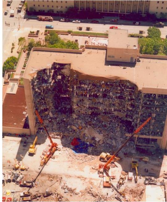
Figure 1.1: Partial collapse of the Alfred P. Murrah Federal Building ( www.fbi.gov )
