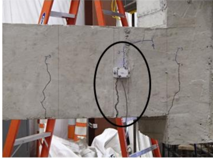
Figure 5.2: Critical flexural crack near the center column (Specimen 1)
