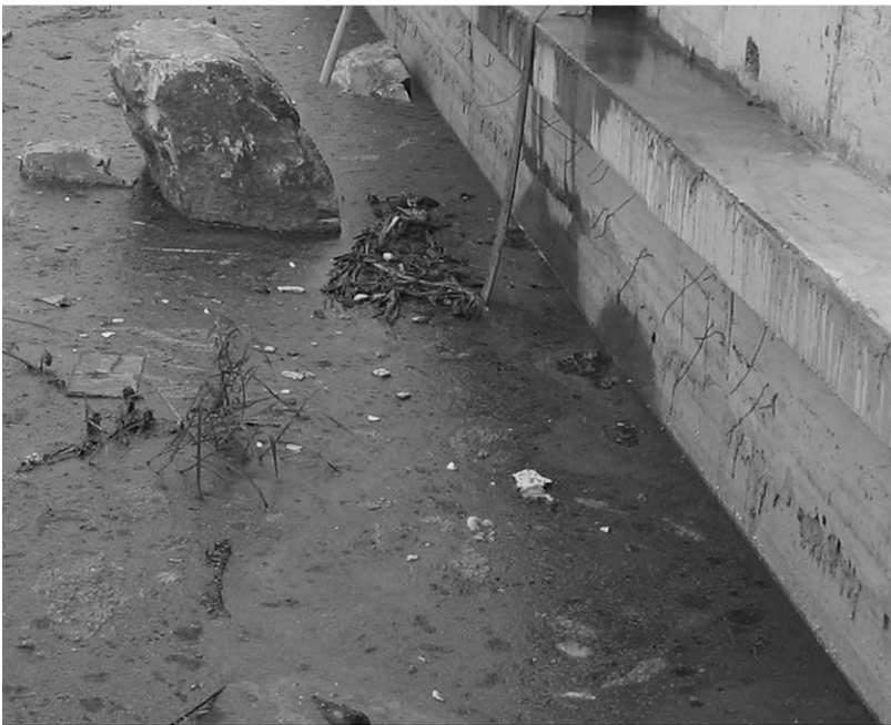
Figure 3. Existing conditions of the canal were quite challenging
