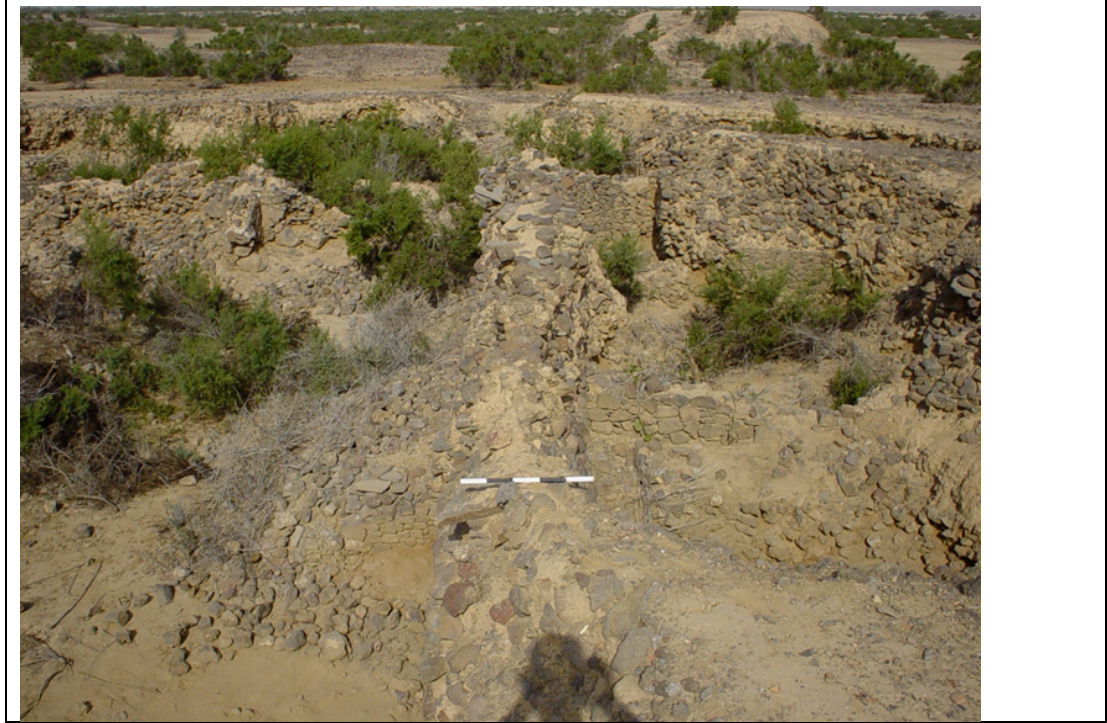
Figure 301 Built form 8 current status, Deteriorating excavation pit for being left for open. Image Source DH
