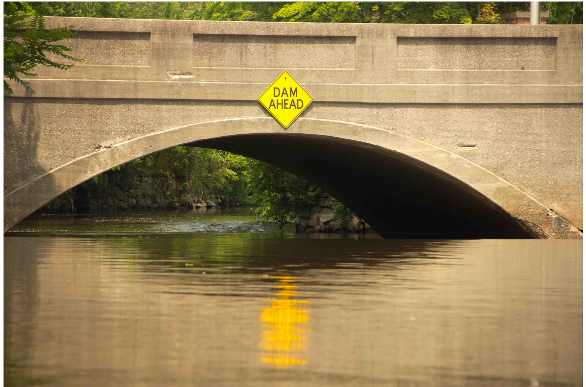
Figure A.1. Some dams in Massachusetts feature warning signs to alert those upstream of the dangers ahead. Many do not, however.
