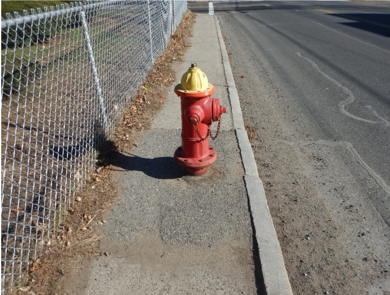
Figure 135: A fire hydrant along McKinstry Avenue
