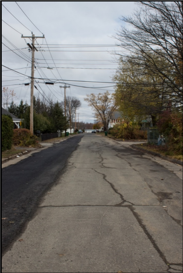
Figure 58: An example of deferred or poor maintenance in Aldenville
