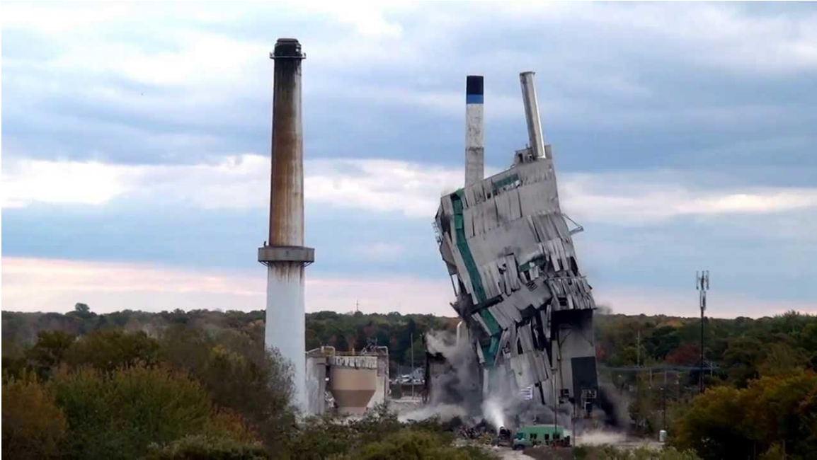
Demolition of paper mill on the Muskegon Lake south shoreline Still frame from video (Race, 2013)
