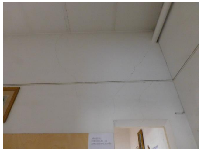
Figure 8. Widespread cracks having width smaller than 3 mm. First floor, wing on piazza Verdi
