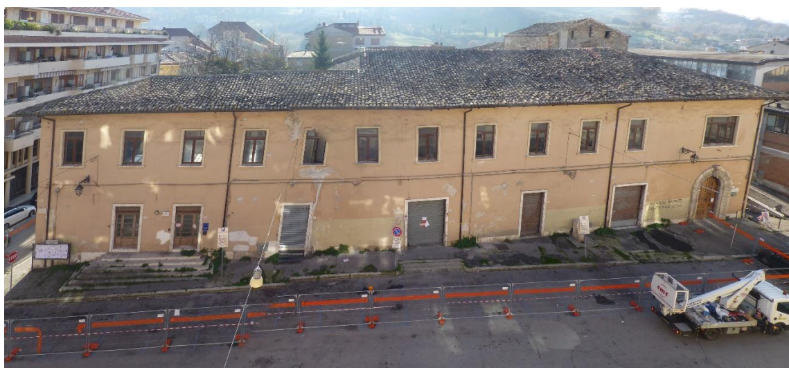
Figure 5. Photomerge of the façade on piazza Verdi (Figure 1) and related roof after the October 30 th event
