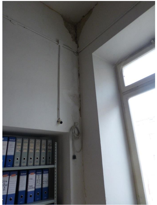
Figure 12. Separation between partition (left) and structural wall (right). First floor, room on piazza Verdi
