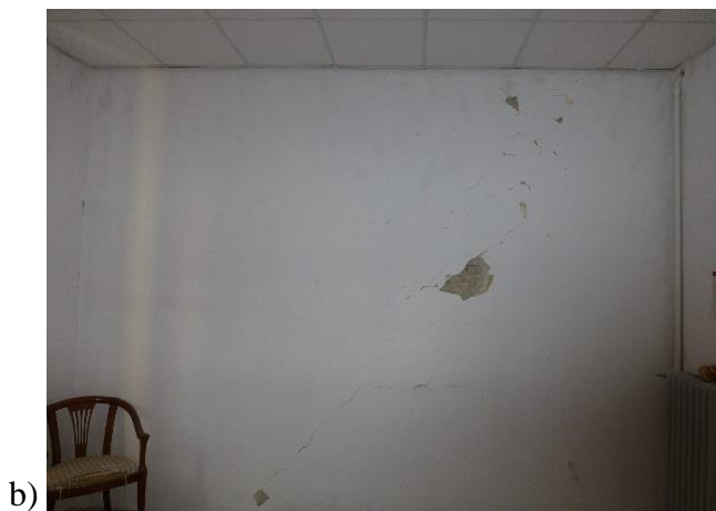
Figure 11. Inclined cracks crossing the whole thickness of a partition between two rooms on via Cameli garden
