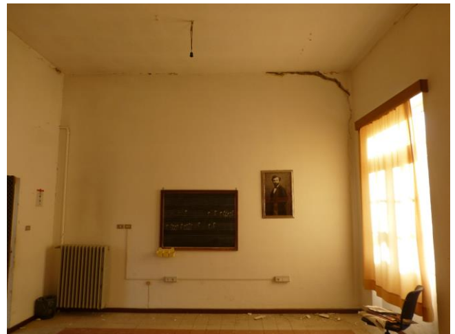
Figure 9. Evident separation between vertical and horizontal structures, as well as at wall intersections. First floor, wing on via Stazio
