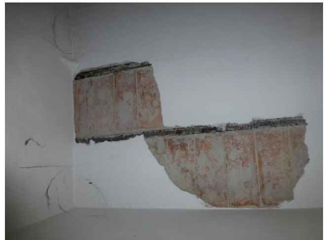
Figure 13. Plaster delamination from intrados of I-beams and hollow clay blocks floor. Ground floor, room on via Stazio
