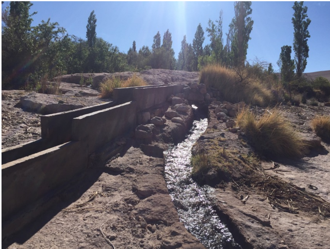
Figure 5.11 | Different types of infrastructure
