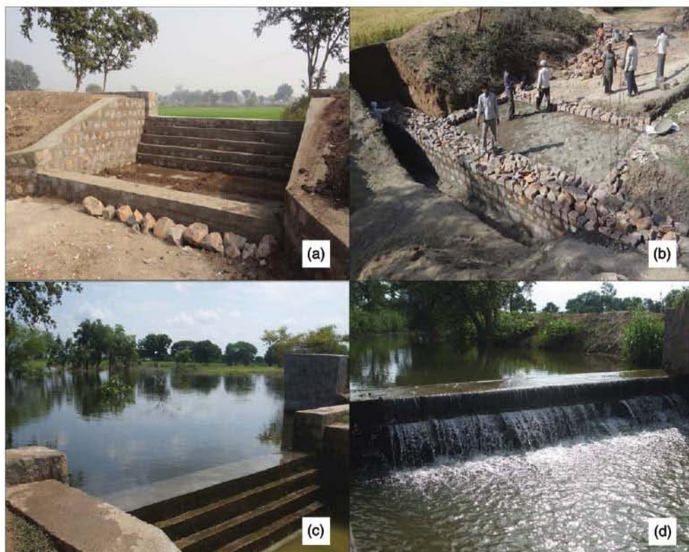
Fig. 7.5. Rainwater harvesting in watershed: (a, b) check-dams constructed at different locations; and (c, d) water harvested in check-dams during the rainy season 2013–14.
