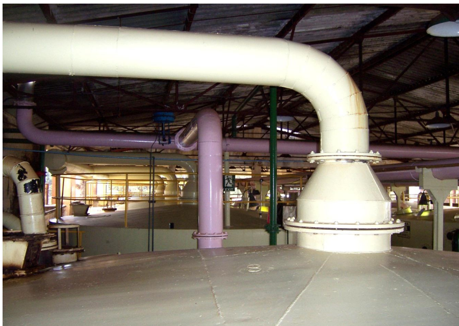
Figure 17: Fermenters of a sugar cane bioethanol plant, Brazil (© Rutz)
