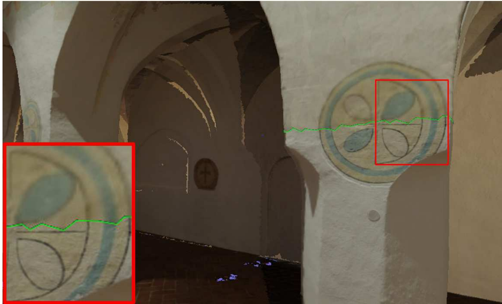
Figure 3.25. Model textured with distant images, while a close up image brings significant improvement in resolution, as seen on the bottom part of the pillar. Green line marks the texture boundary.
