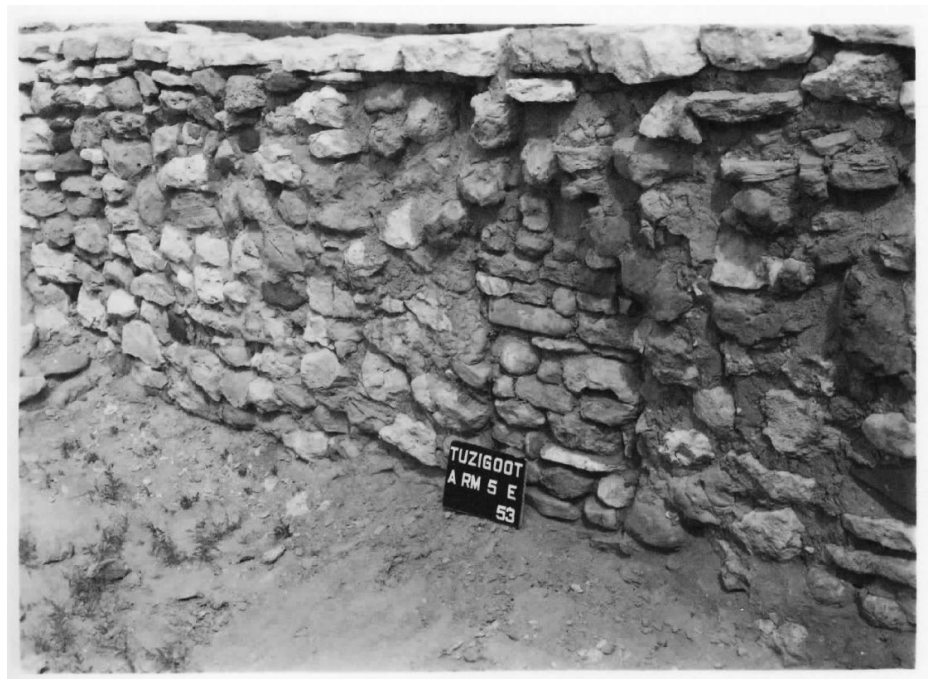
Figure 40 / Photo of wall 4C (east wall of room III-5) after stabilization completed by Richert in 1953. The work completed involved clearing the wall out, grouting it with cement, and masonry facing was pointed with soil cement.
