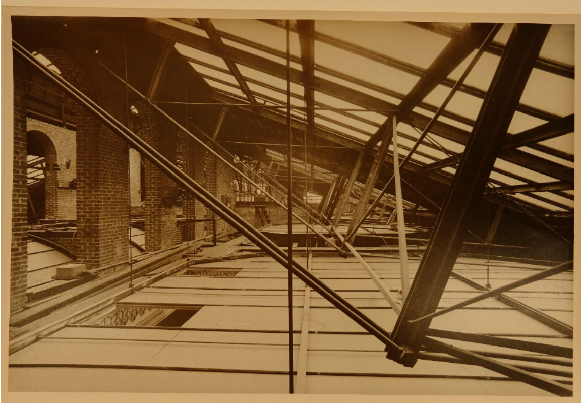
Figure 16 Detail of the skylight structure (North side of the museum) (Harris Davis Photography 1973)
