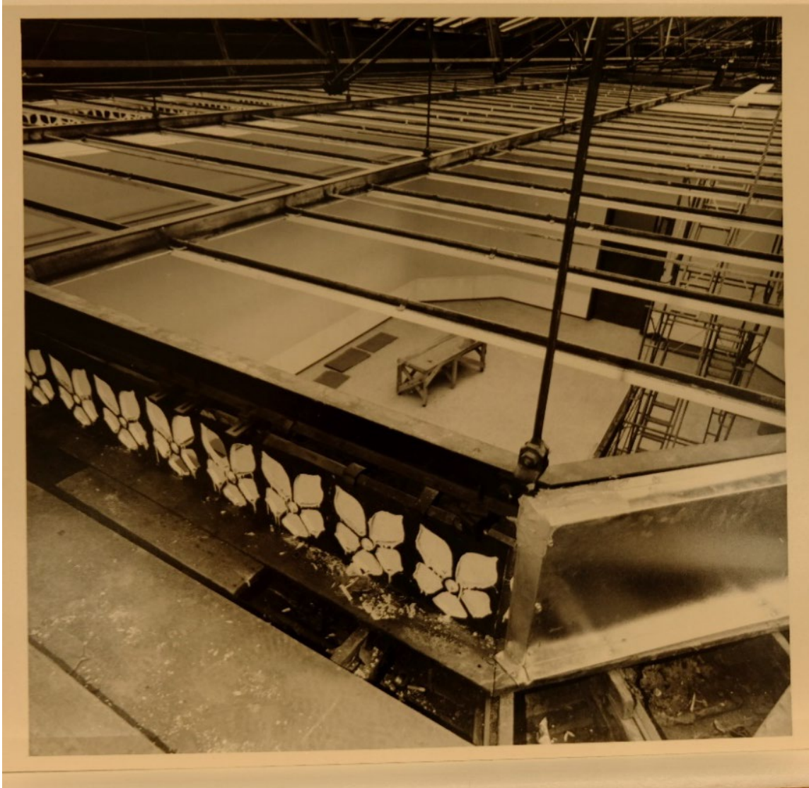
Figure 19 Detail of the skylight structure above the gallery space (Harris Davis Photography 1973)
