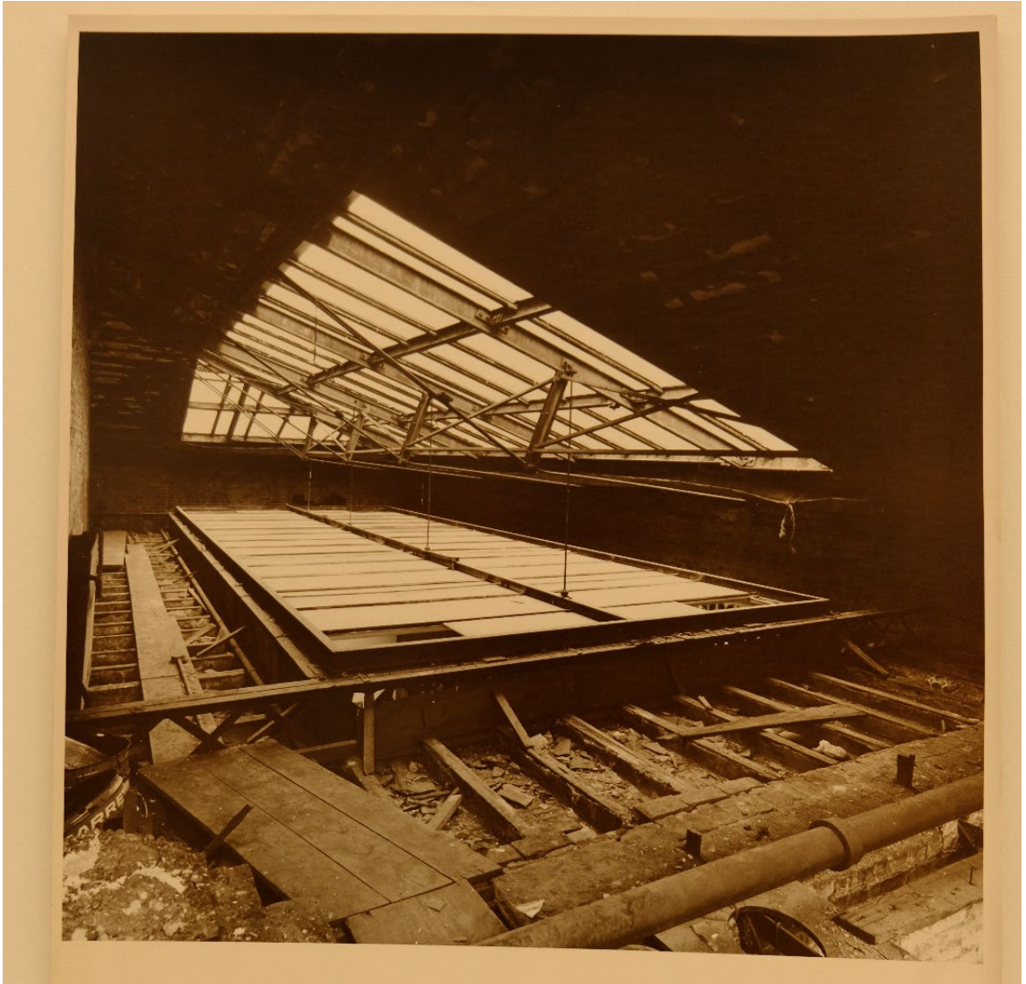
Figure 17 Detail of the skylight structure (North side of the museum) (Harris Davis Photography 1973)
