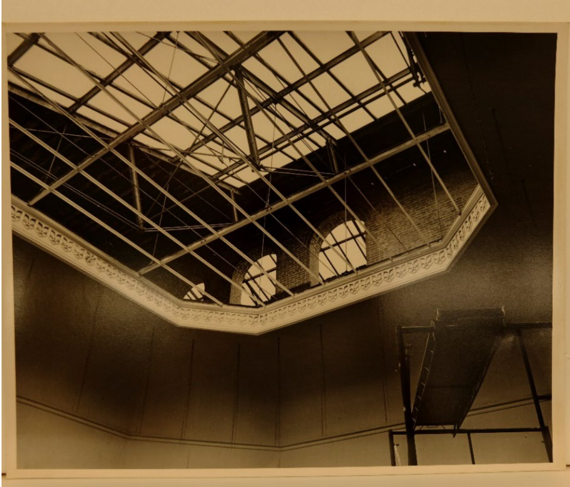
Figure 18 Detail of the skylight structure (view of skylight frame from the gallery) (Harris Davis Photography 1973)
