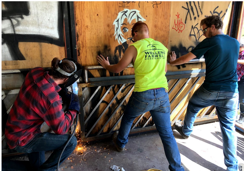
Severin Elste welding a railing to the steel mullions while Chris Levy and Karl Wellens holds it in place
