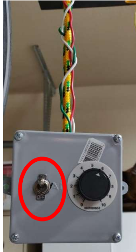
Figure 3. Emergency switch location
