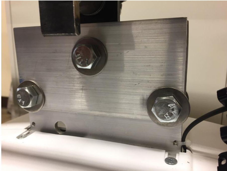
Figure 27. Hanger bracket, securing Handicare hoist to trolley beneath the I-beam.
