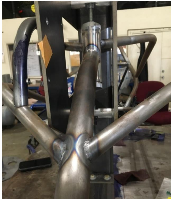
Figure 57. Middle and top side supports full welded, in progress welding the mid-drive truss members.
