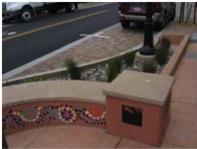
Figure 11: Seat wall and stormwater planter Source: Guide to the San Francisco Better Streets Plan
