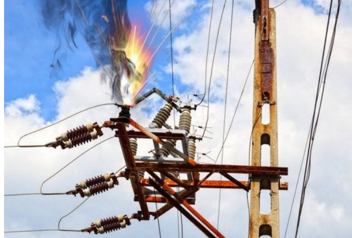
Figure 1.1: Example fault in a power line detectable through the use of relays [2]
