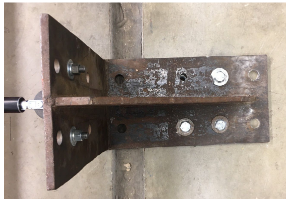
Figure 3.1.2 The angled base plate that holds one end of the damper through a pinned connection, anchored into the floor slab with 3/4" bolts.
