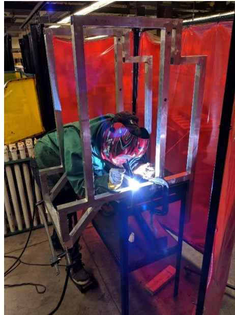
Figure 36. Welding the cross members to join the two sides of the frame together.
