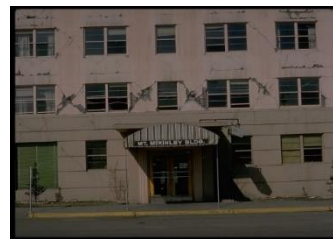
Shear Damage Short Column
