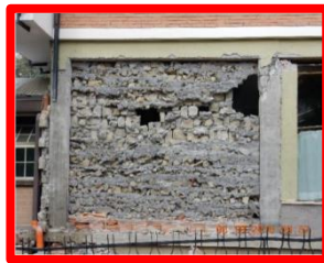
Infill Collapse RC Frame
