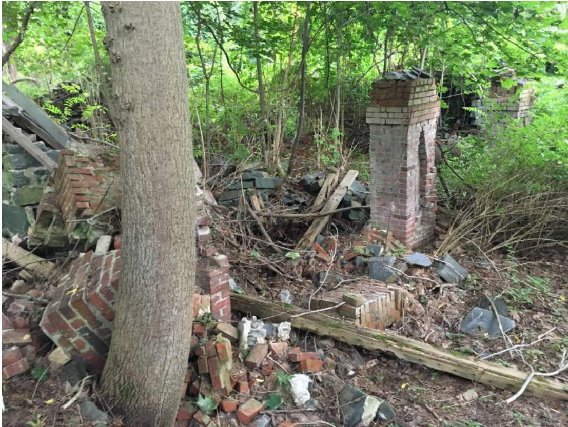
Figure 25: The crumbling foundation of Vassaar's Cottage. The brick pillars can be seen in Downing's drawing of the rear elevation (figure 6)
