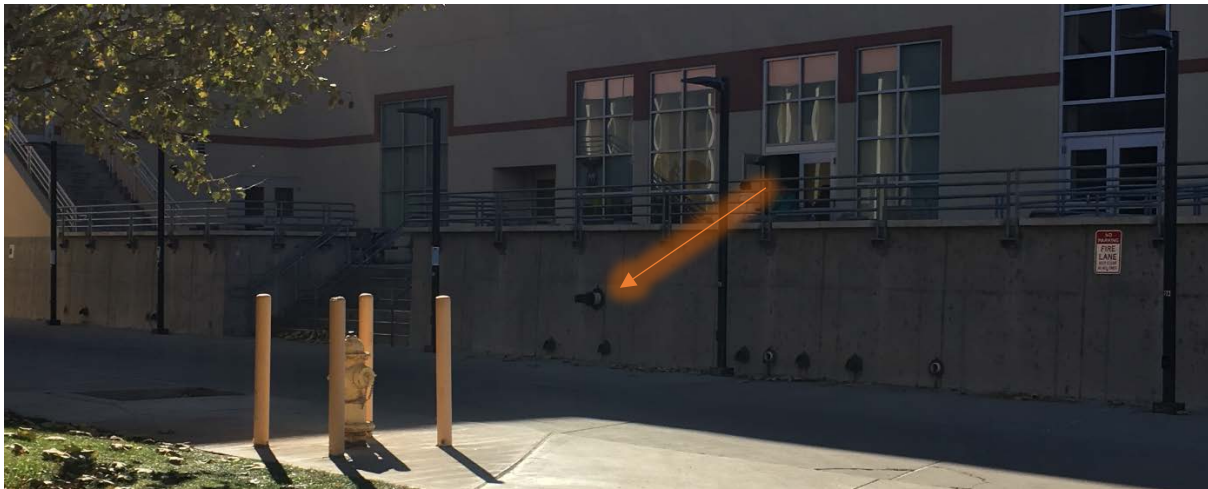
Figure 5-2 - Fire Department Connection
