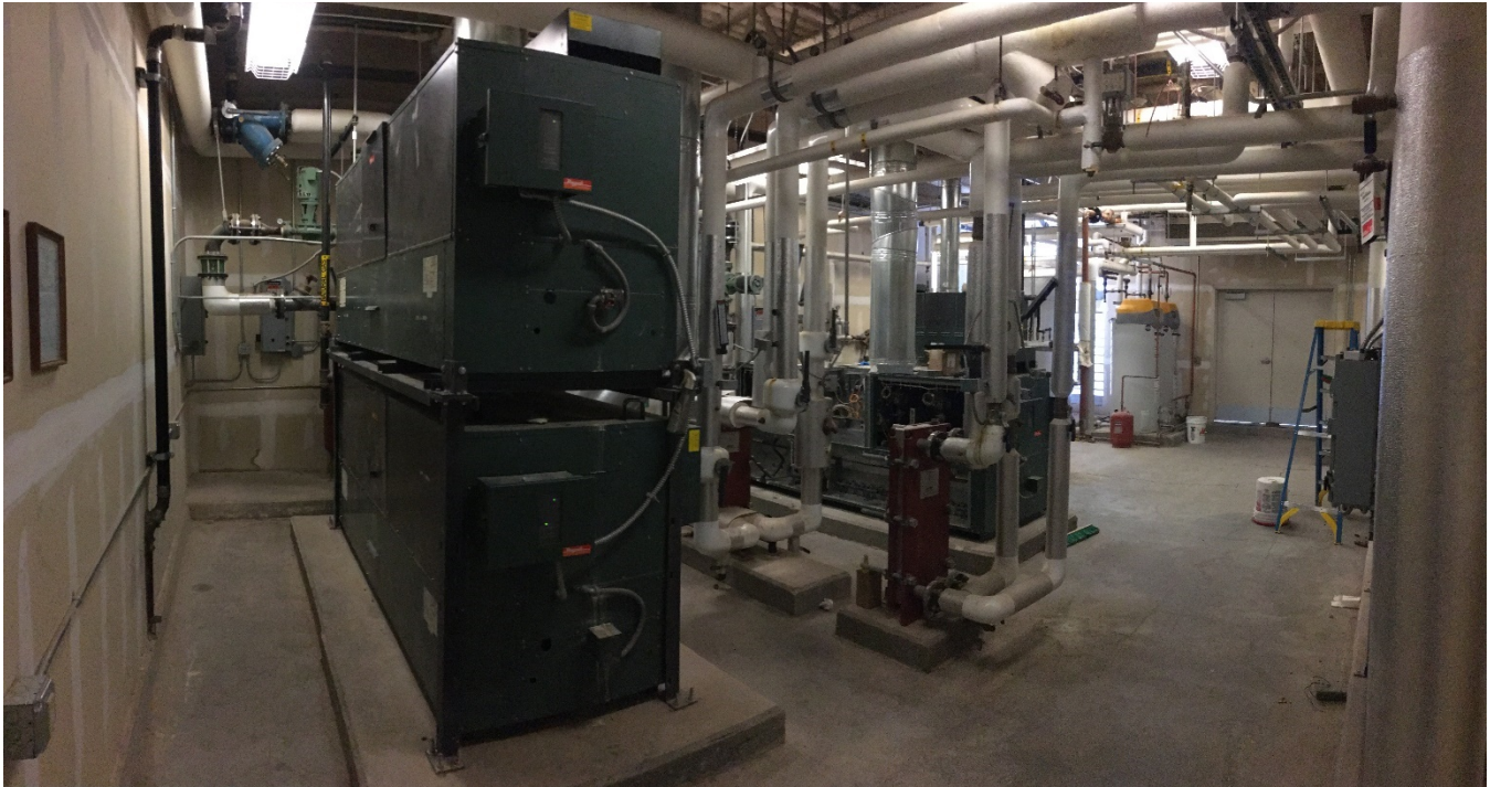
Figure 8-7 - 4th floor Mechanical Room
