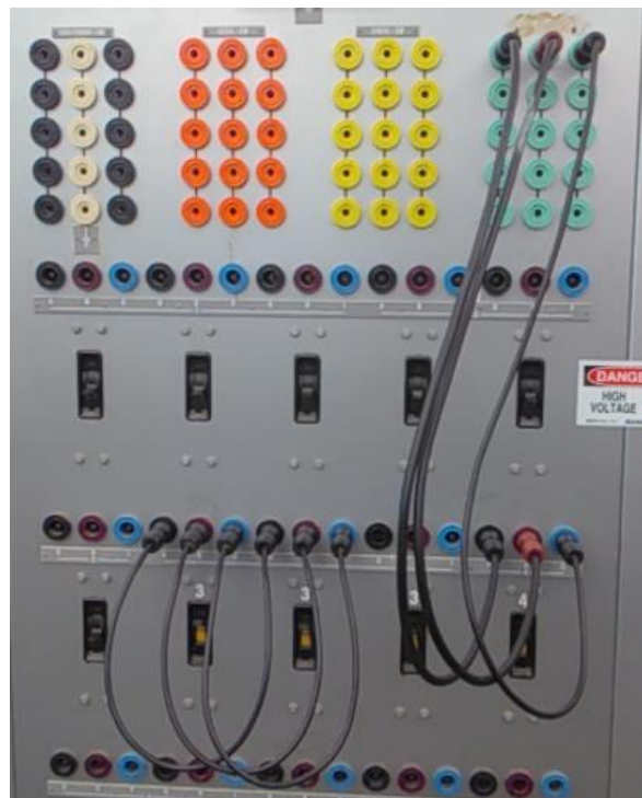
b) Main Distribution Panel Connections
