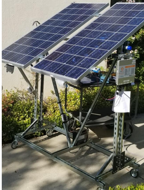
Figure 11. Solar Panel Cart (Troy) and APsystems Microinverter Used in the Testing
