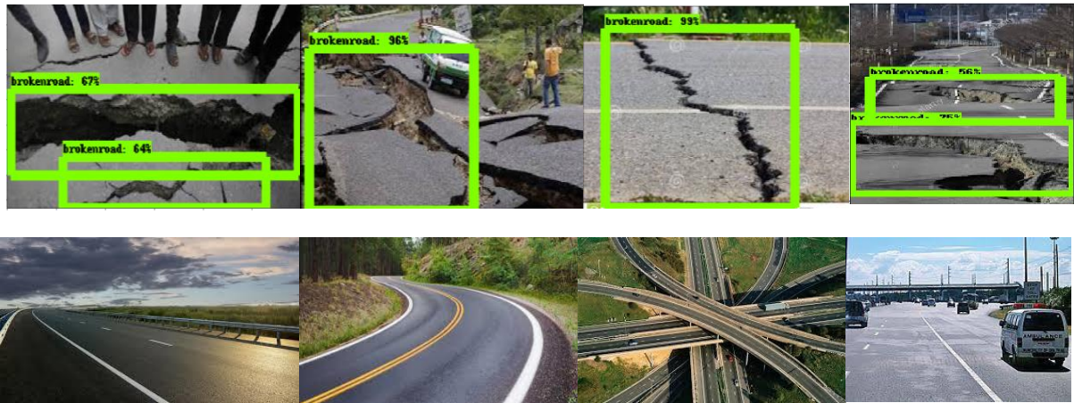
Figure 7. Output images from deep learning classifier for the set of images from Figure 6. Note: If the algorithm does not detect damage, the original image will remain unchanged as seen with images of no cracking.
