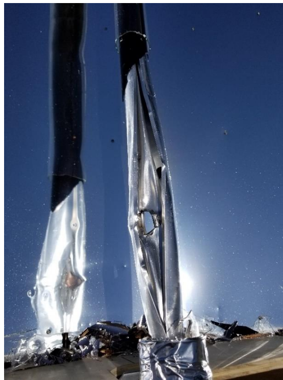
Figure 4.7: Broken Evacuated Tube
