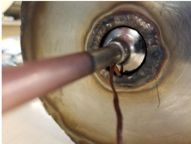
Figure 3.46: Boiler Manifold Plug with Heat-Pipe Bulb and Thermocouple
