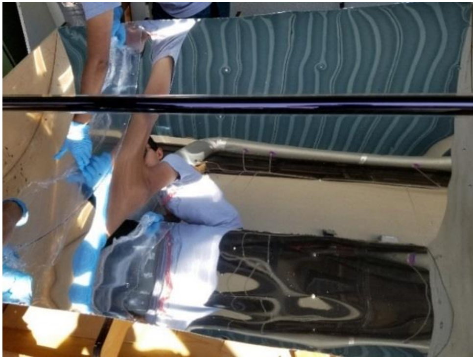
Figure 3.28: ReflecTech® Final Application
