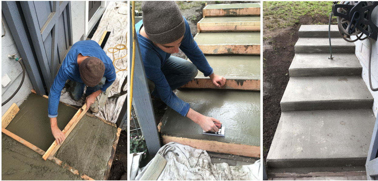
Fig. 4: Screeding over concrete Fig. 5: rounded off corners w/ edger Fig 6: finished product
