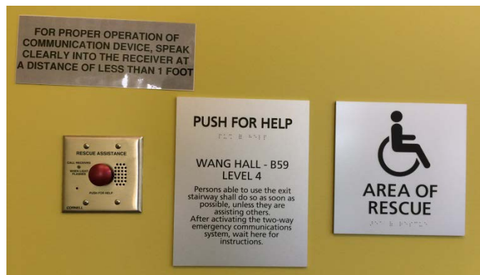
Figure 29: Area of Refuge Emergency Communication Device
