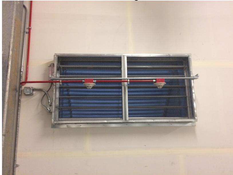
Figure 17: Electric Room Damper Smoke Detectors
