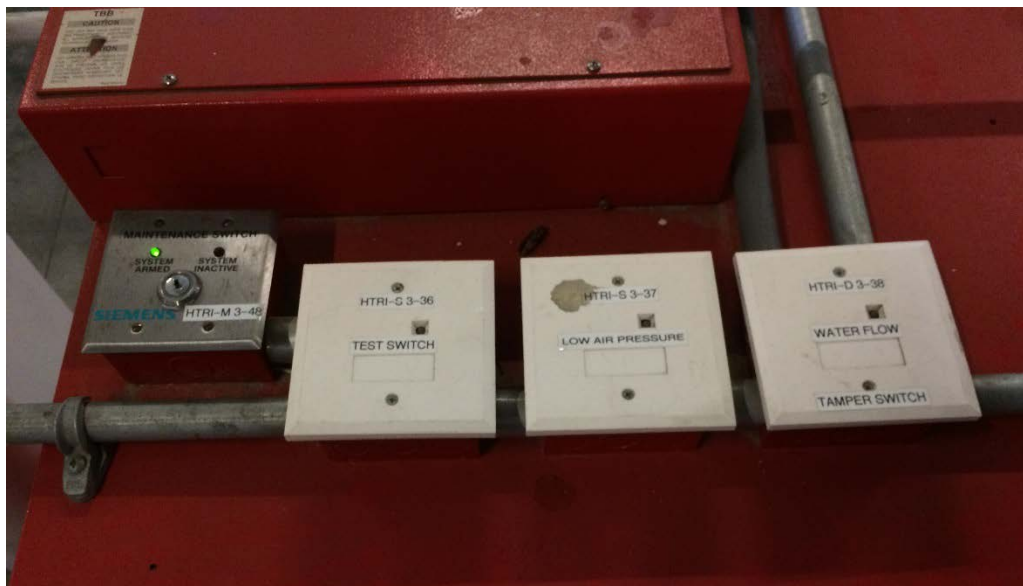
Figure 23: Preaction Sprinkler Monitor Modules
