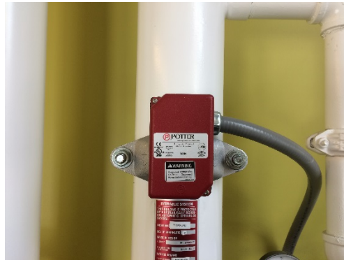
Figure 21: First Floor Water Flow Switch
