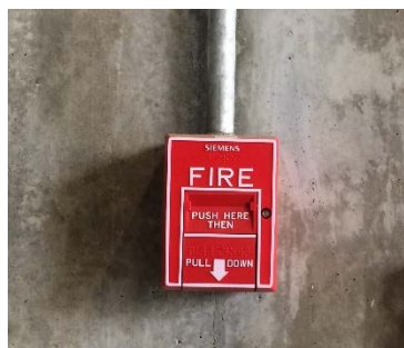
Figure 14: Manual Fire Alarm Box
