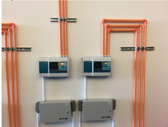
Figure 19: Computing Level VESDA Control Units
