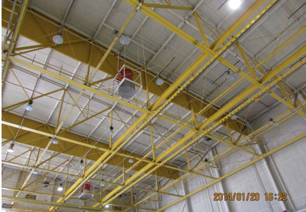
Figure 6-32: HEF Foam generators. (Note the smoke curtains separating the wet pipe systems)
