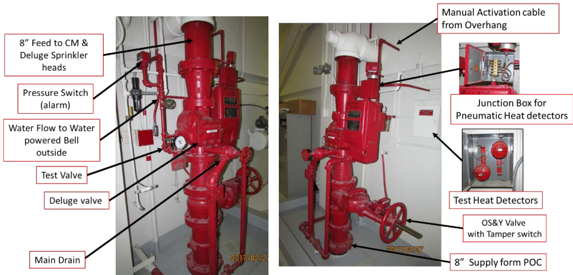
Figure 6-19: Photograph of Riser 2 and the test heat detector
