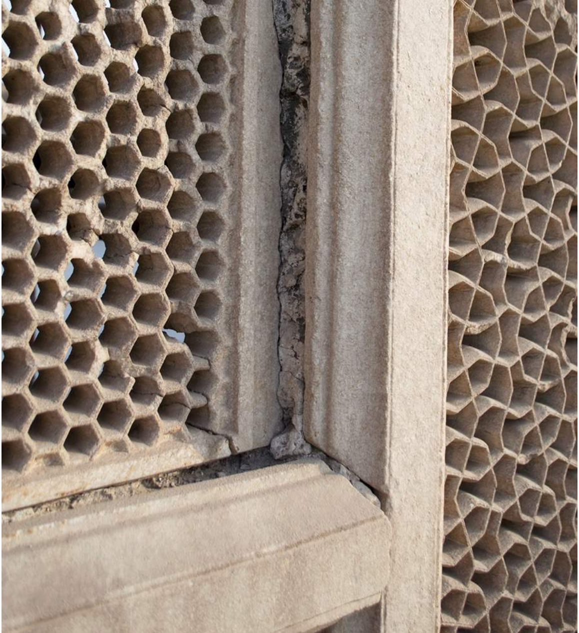
Figure 33: Displacement of the marble jali as it tilts along the façade due to thermal movement.
