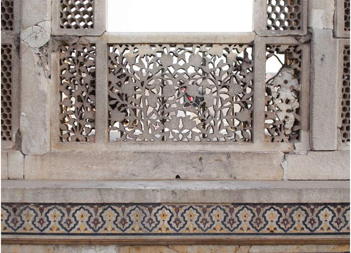
Figure 23: Atmospheric soiling on the central jali of the Naulakha Pavilion.
