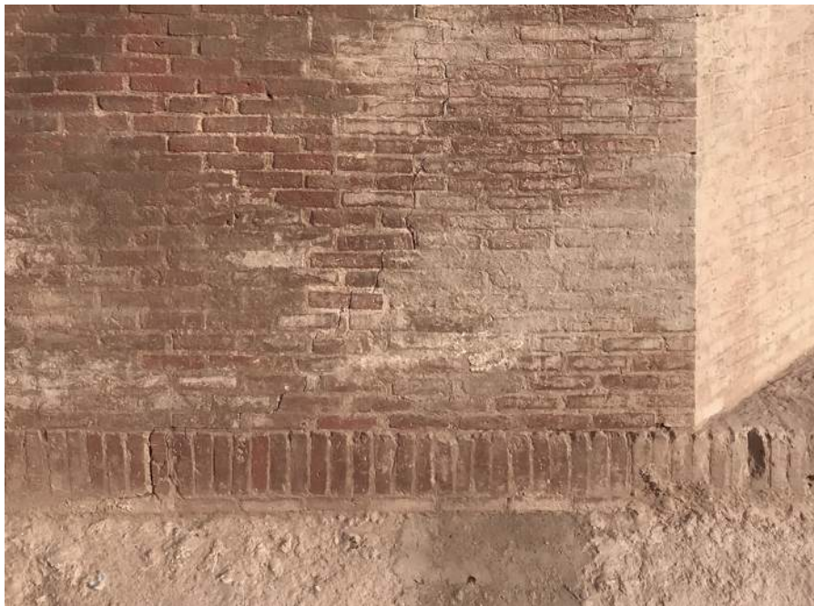
Figure 41: Structural cracks beginning at ground level as seen on the Picture Wall.
