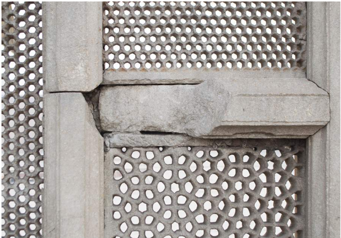
Figure 24: Open joints in the supporting frameworks of the jalīs. Mostly seen as a result of mortar deterioration and spalling.
