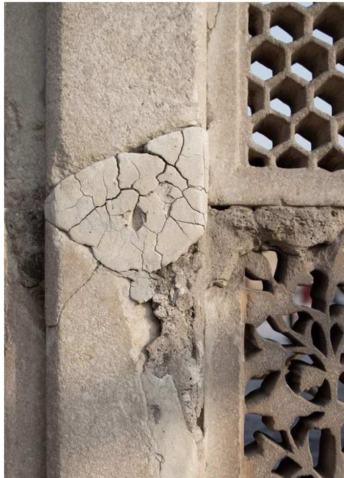
Figure 39: Incompatible marble-dust fill repairs showing extensive network cracking.
