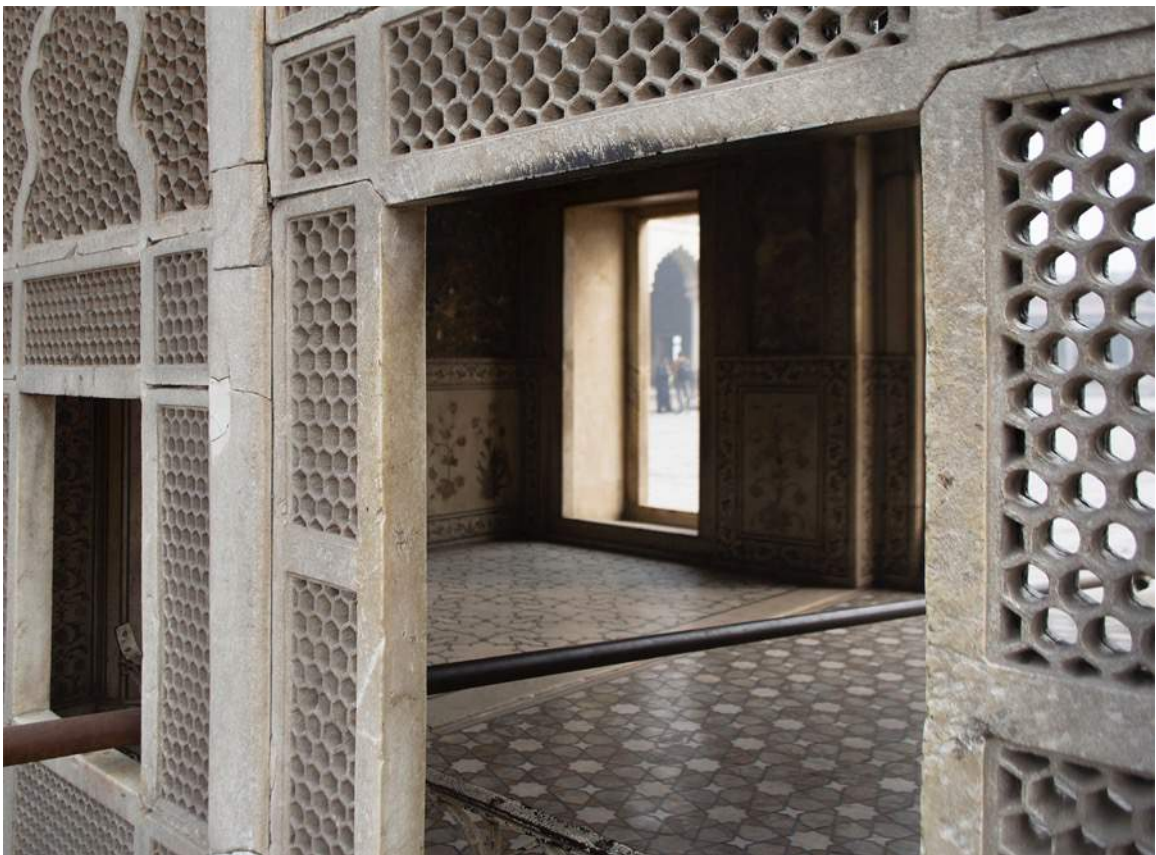
Figure 25: Gypsum related black crust seen on the underside of the central jali.
