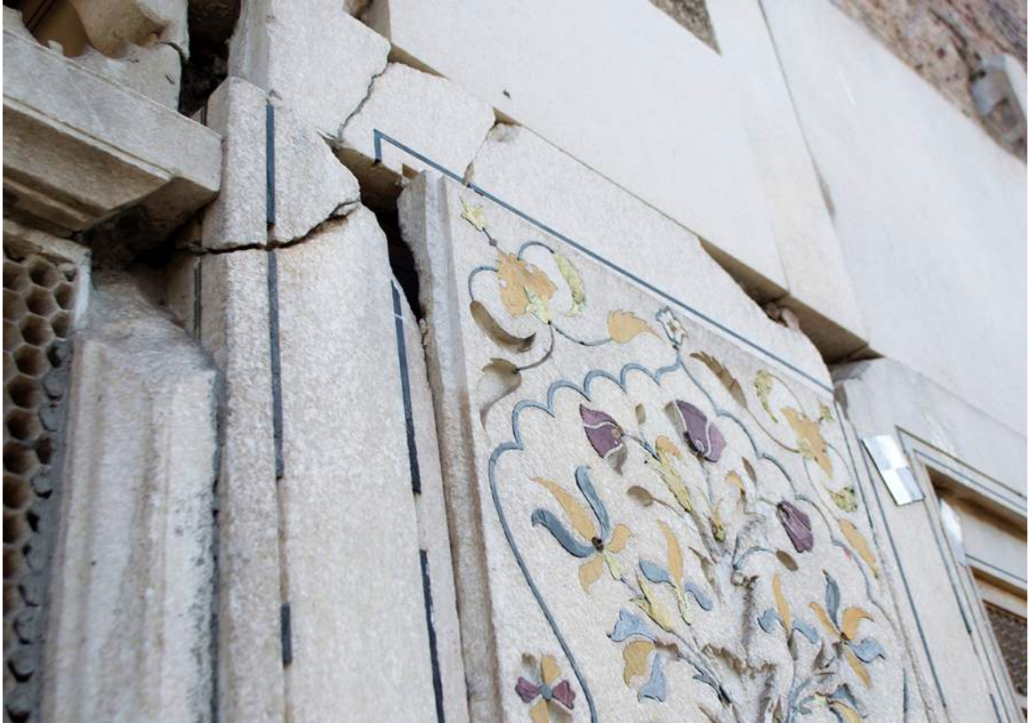
Figure 34: Displacement of the parchin kari (pietra dura) panel as it tilts across the façade.
