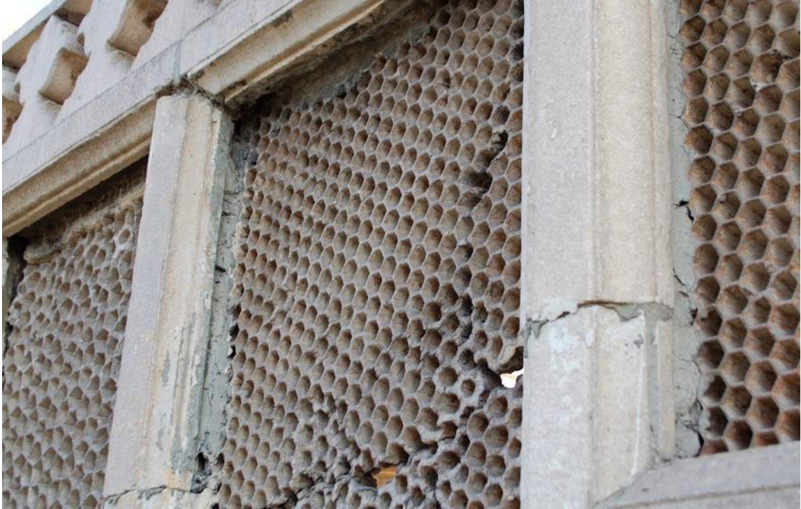
Figure 38: Incompatible cementitious mortar used for resetting the jalis and their frameworks (2000).
