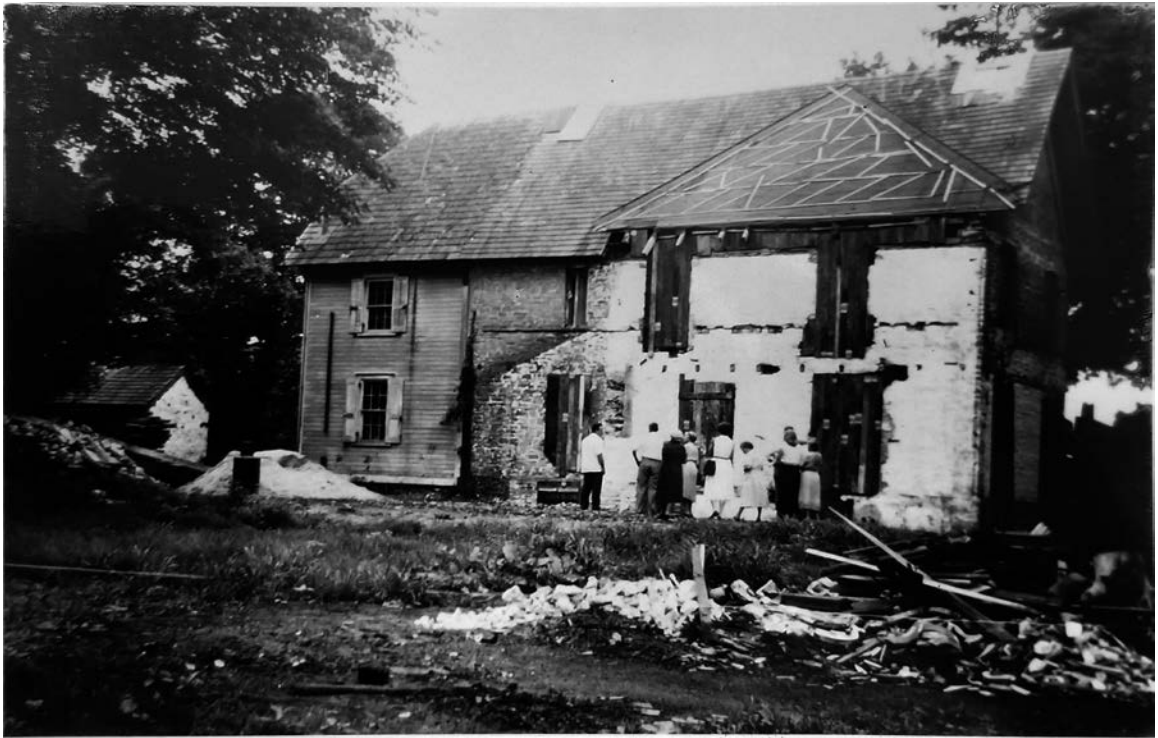
FIGURE 17: North elevation (rear) of the 1704 House during restoration after removal of the serpentine wing. (Image: Clement S. Brinton, 1954, from Photo Archives, Chester County Historical Society)
