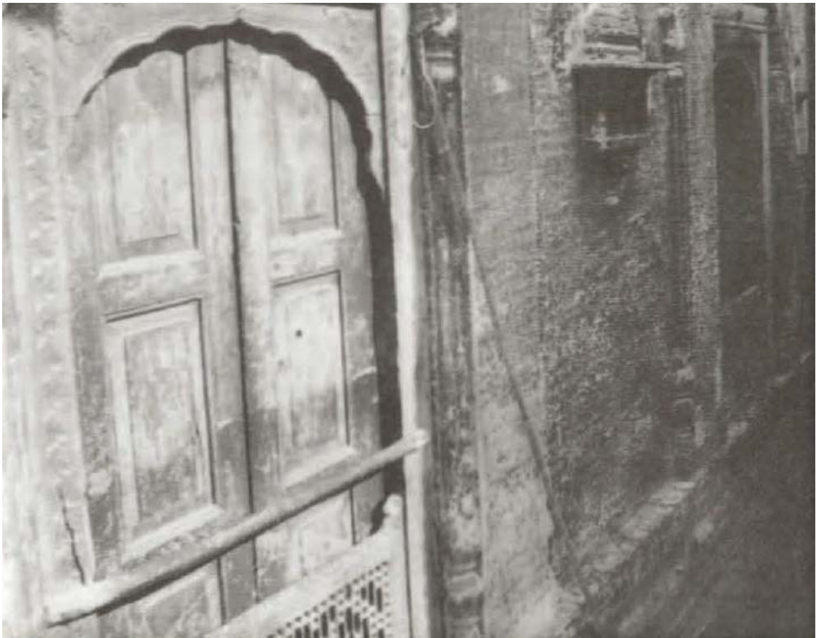
Fig. 35: Window Detail on South Facade of House D/3264 (Source: The Walled City of Lahore, publication by PEPAC)
