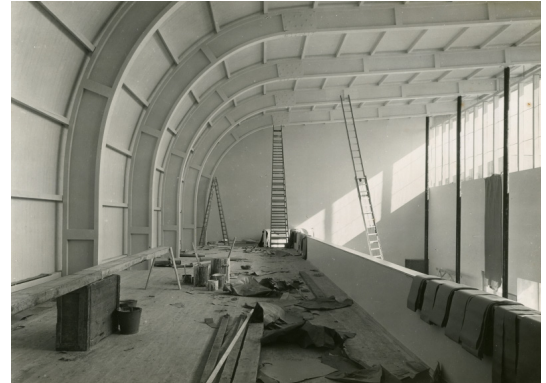
fig. 12, below: Functionalist architecture was enabled by new industrial materials, such as the steel frame, seen here.
