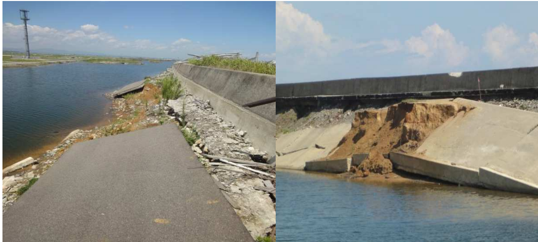
Figure 1.1. Examples of damages caused by the 2011 Great Eastern Japan Earthquake and Tsunami (Jayaratne et al., 2013).
