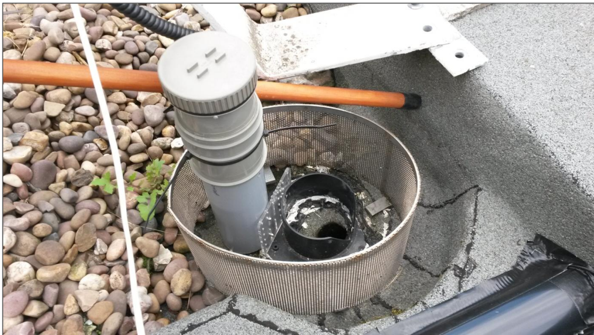
Figure 6. V-notch capacitance sensor monitoring device. (Top) V-notch installation; (Bottom) Capacitance sensor stilling tube attached to v-notch.
