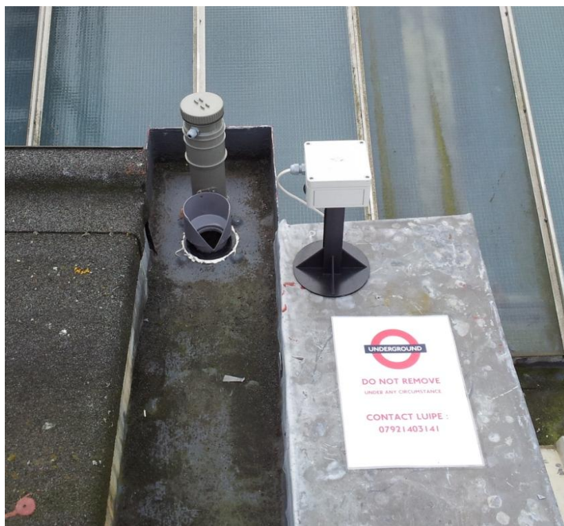
Figure 5. V-notch capacitance sensor monitoring device in-situ on the London Underground depot at Ruislip, London.
