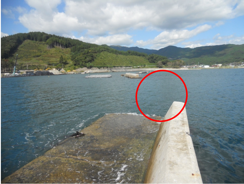
Figure 7. Damaged breakwater at Okirai port, showing missing caisson sections.
