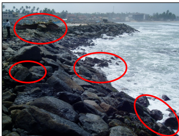
Figure 1. Displaced rock armour at the seaward side of the outer breakwater at Hikkaduwa.
