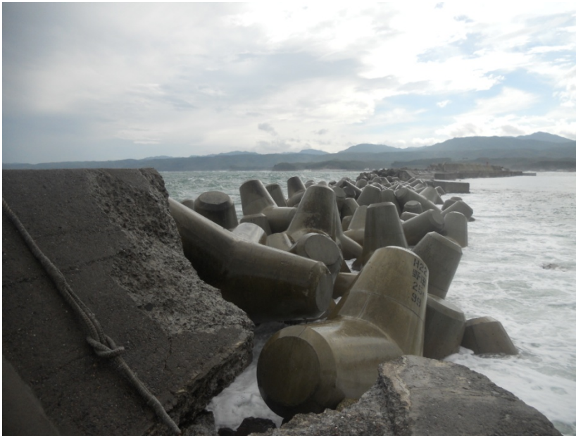
Figure 5. Damaged Breakwater at Noda Port, provisionally repaired using 25 ton tetrapods.
