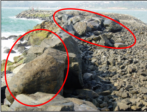
Figure 3. Displaced primary rock armour at seaward and crest of the main breakwater at Puranawella
