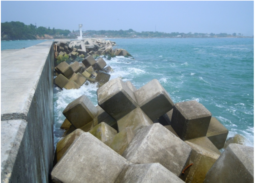
Figure 10. Failed X-Block Armour Units at Hikado Port.
