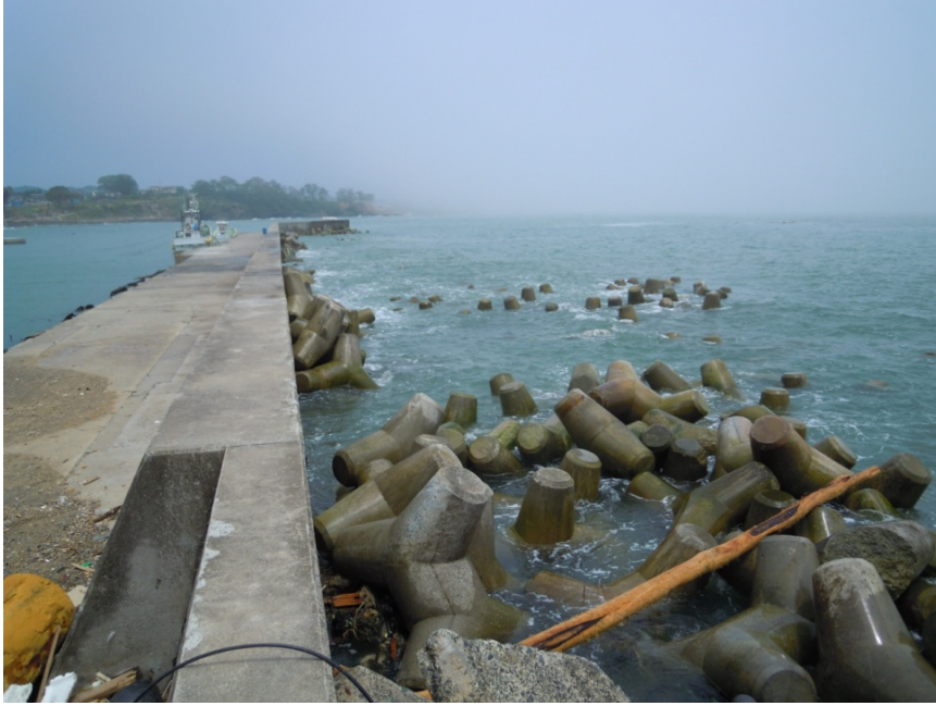
Figure 9. Damaged Sea-Lock Armour Units at Ooya Port.
