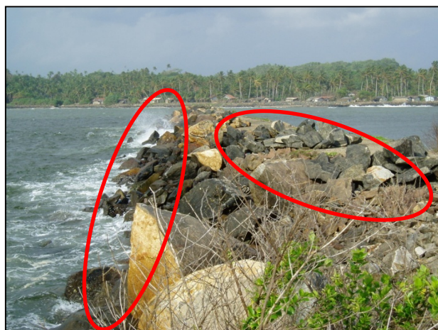
Figure 2. Displaced primary rock armour at the seaward and crest of the main breakwater at Mirissa
