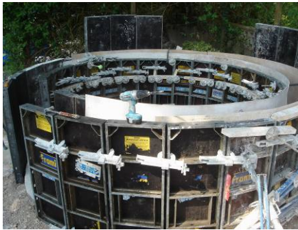
Figure 1: Concrete formwork for rammed chalk - Calyx visitor centre, Dover 2007 by Rowland Keable
