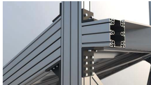
Figure 5 – Staircase beam and bottom chord connected to portal frame using angle plates
