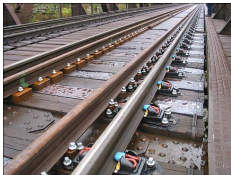
Fig.6. Installed fastening system with ZLR clips (Pandrol VIPA system) on a bridge
