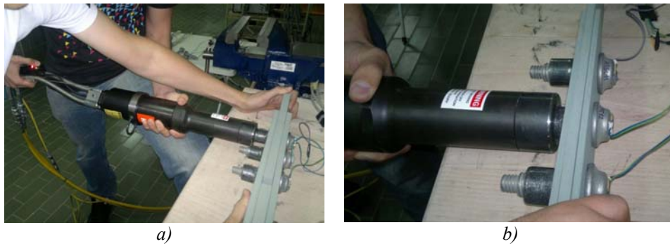
Figure 6. Installation procedure of Huck BobTail bolts diameter 20 mm: a) red light indicates that the tool is activated b) close-up view
