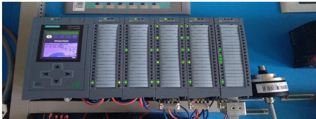
FIGURE 2: S7-1500 PLC WITH HIGH-SPEED COUNTER
