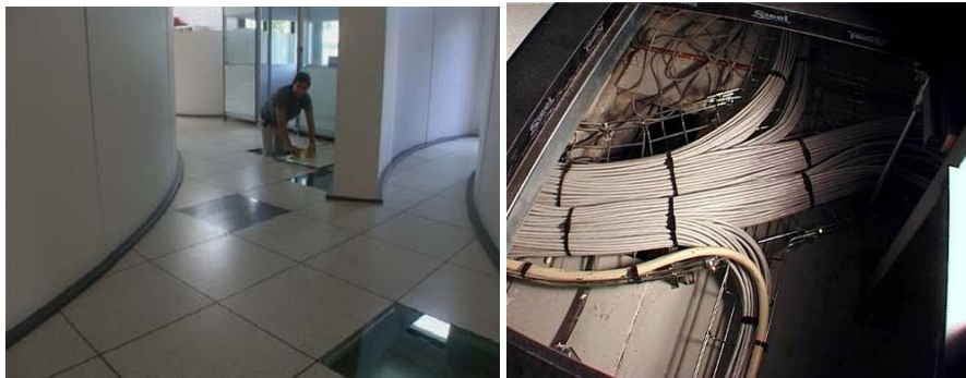
Figure 5.9. The infrastructure of K1 Building: raised floors. Left: a user moves a tile with a suction grip. Right: the “highway” of network cables as they originate from a control room and run to underfloor distribution boxes in various areas of the building, where local cables with a loose end can be plugged.
