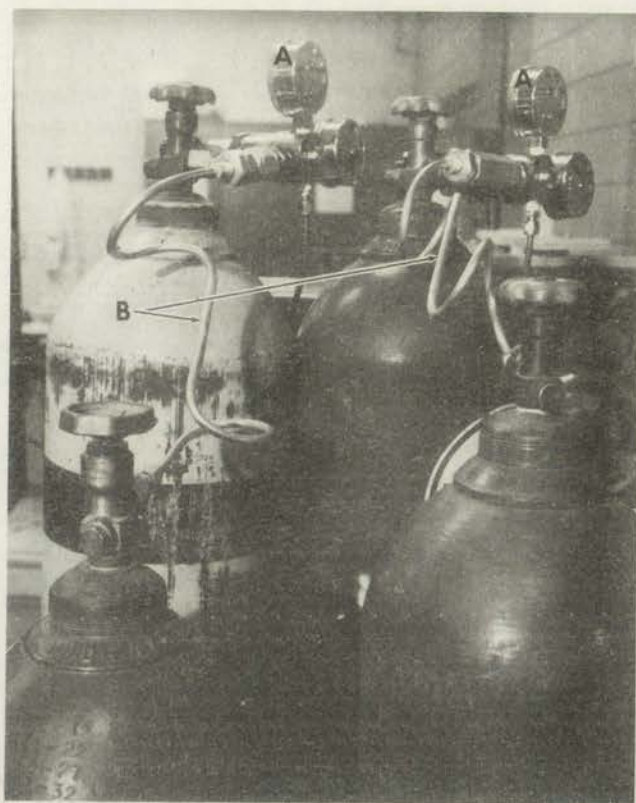
Figure 7. (A) High Pressure Regulator (B) Manifold System
