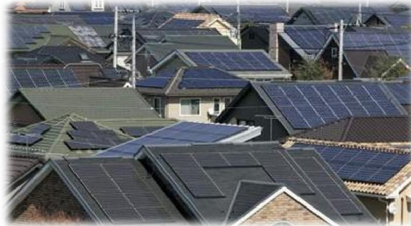
Distributed Solar PV
