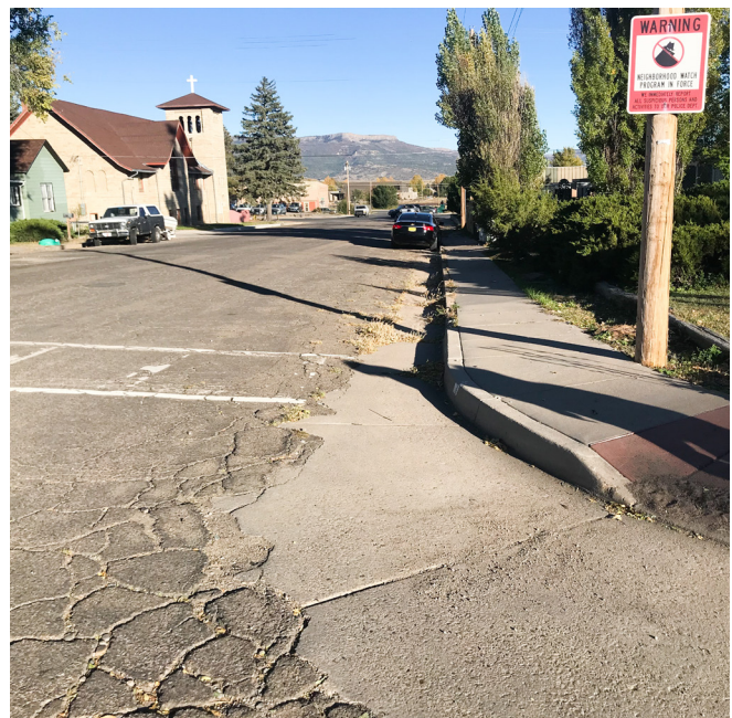
A faded crosswalk at Apache Ave. & S. 3 rd St.
